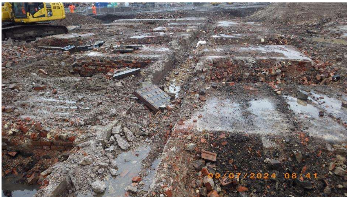
NT02: buried obstructions
