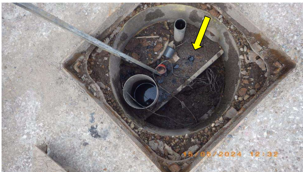
NT03: single chamber interceptor, close to bend in MP gas main (see Section 4). Liquid contents clean, small 'tide' mark of slightly impacted material (yellow arrow)
