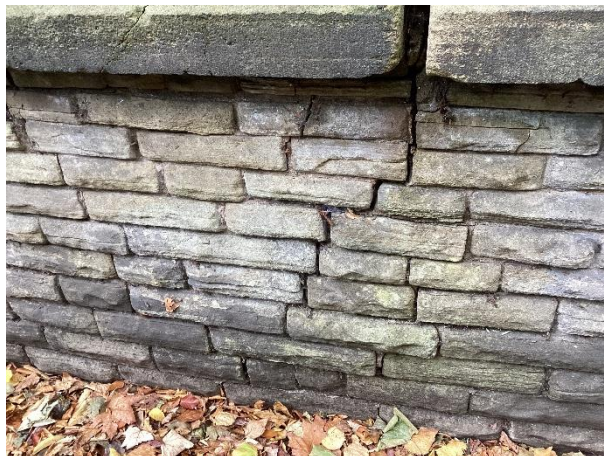
Damage adjacent to chestnut tree
