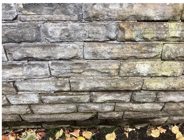
Severe lean adjacent to the lime
