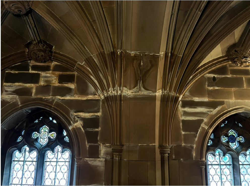
3.13 Internal - Signs of Water Ingress
