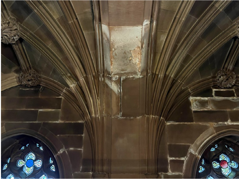
3.12 Internal - Signs of Water Ingress
