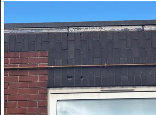
Photo 5 (08/07/2025): Gaps in the brickwork identified on the eastern aspect of the building, found to be superficial on closer inspection with a high-powered torch.
