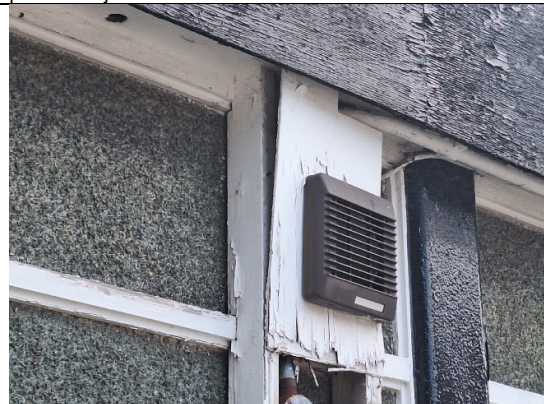
Photo 6 (08/07/2025): Example of a gap in the wooden cladding on the western aspect of the building. Feature fully inspected with a high-powered torch and found to be shallow and limited for roosting bats.
