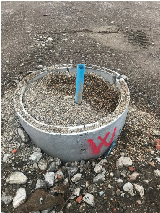
Example 3 : Concrete manhole rig enclosure
