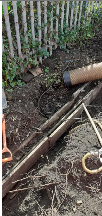
Cables exposed adjacent railway boundary in concrete trough
