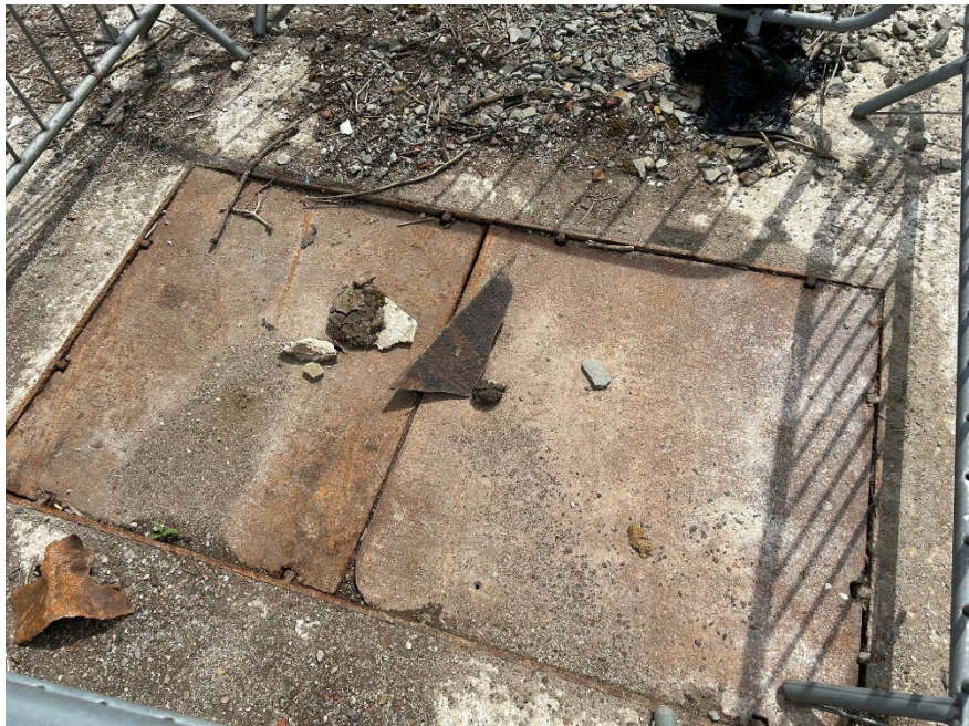
Tank LFT02 Cover
