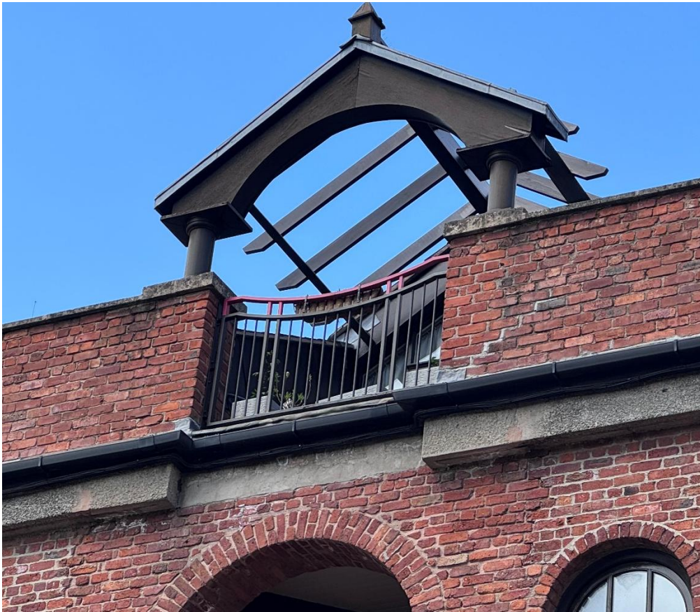
Figure 26: A view looking up at a 1980s dormer balcony to the eastern and of the south elevation, showing the modern recessed guttering fixed to the 1920s reinforced concrete ring beam, and plywood gable structure.
