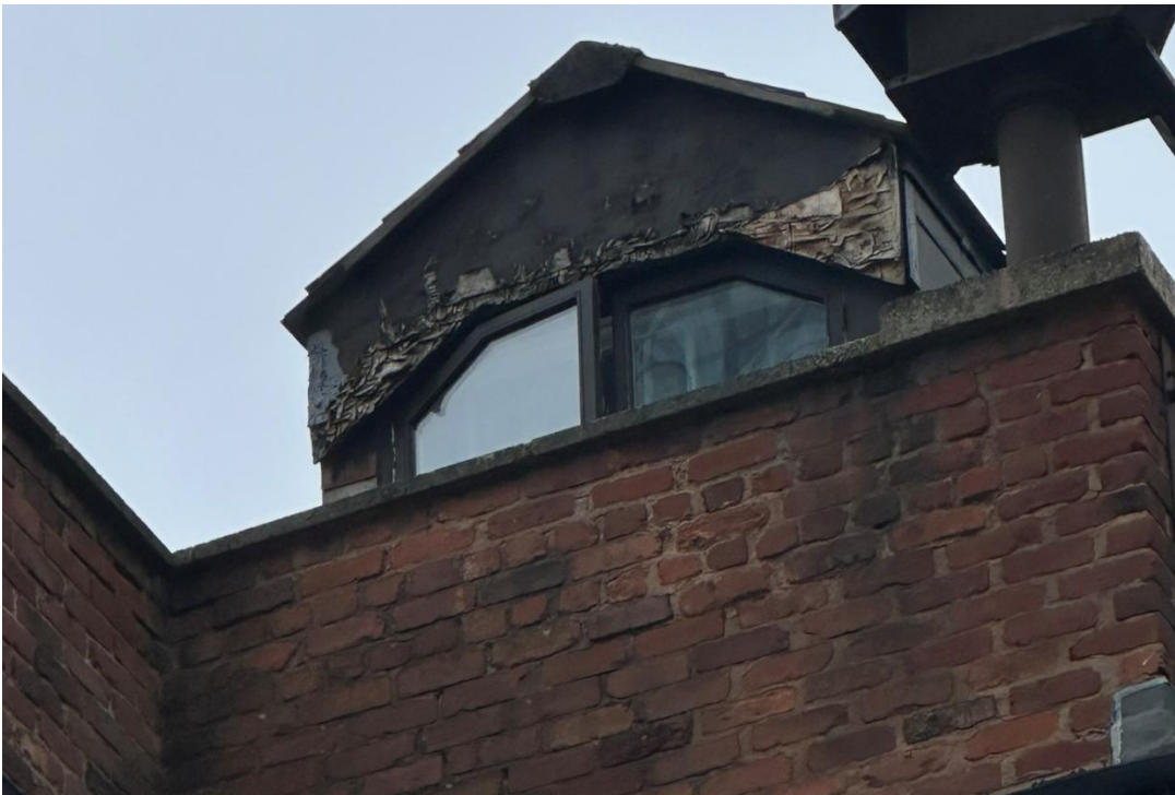
Figure 20: A view of the 1very poor condition of the 1980s plywood fascia board to the dormer window at the south-east corner of the roof level.
