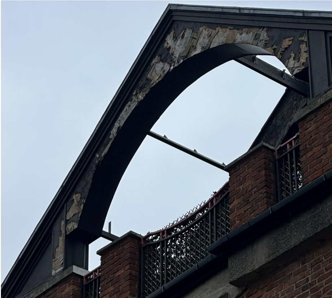
Figure 21: A Similar view to the centre of the south elevation, again illustrating the failure of the original 1980s works to the building.
