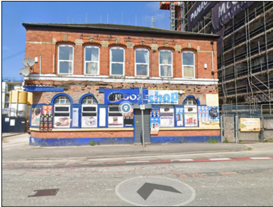
Photograph 9; As much of Rochdale Road was blocked off, a photograph of the lower level from a distance was impossible and a snippet from Google maps has been used to annotate. Gaps along the first storey, front face of the building was noted, these were hollow due to previous exterior fittings.
