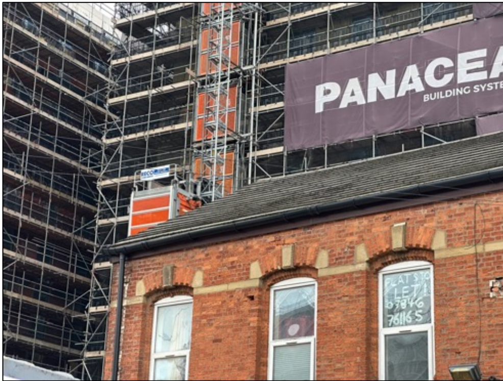
Photograph 3, A front view of the building on site. The external roof is in good condition, fascia boarding was in fair condition along the upper front. Small openings were noted across the upper front face among the brickwork but were seemingly hollow, created by previous fittings.
