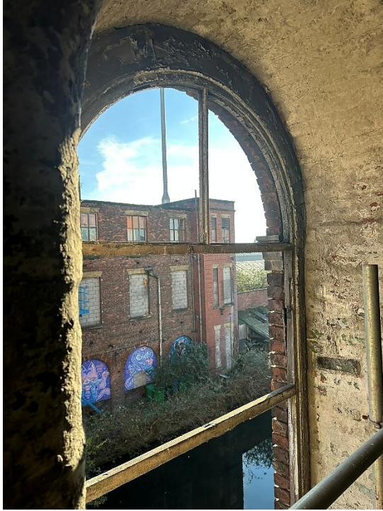
Figure 22 – One of the three southern windows, showing the remains of its original timber casement windows.
