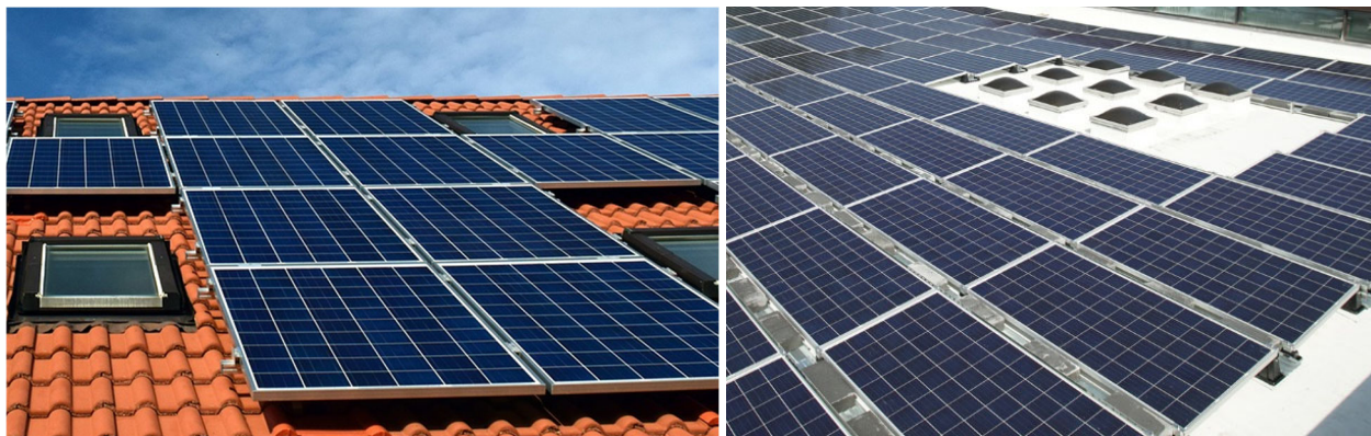
Figure 8 Example SPV array installations
