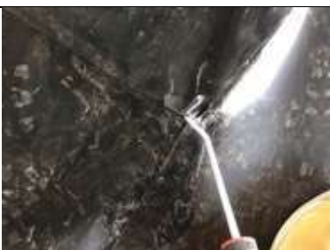
Recorded weld defect
