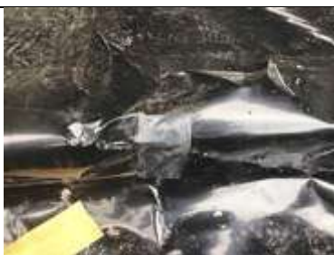
Recorded weld defect repair
