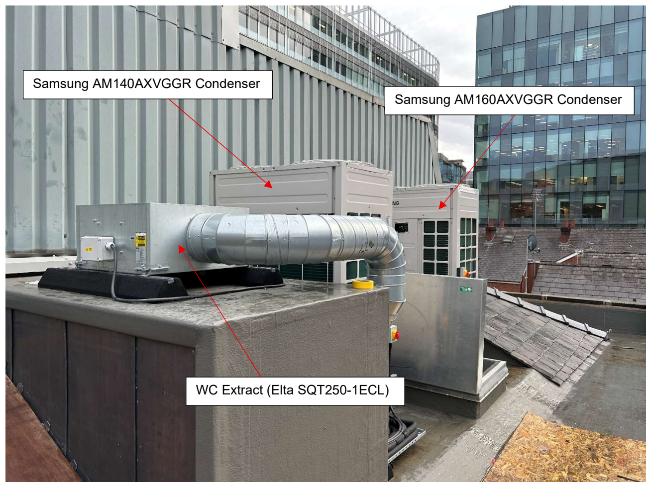
Figure 1 – Rooftop Plant Compound
