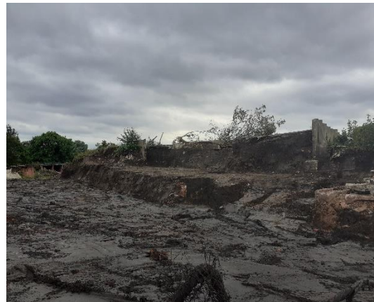
Photo 22: Banking area complete
