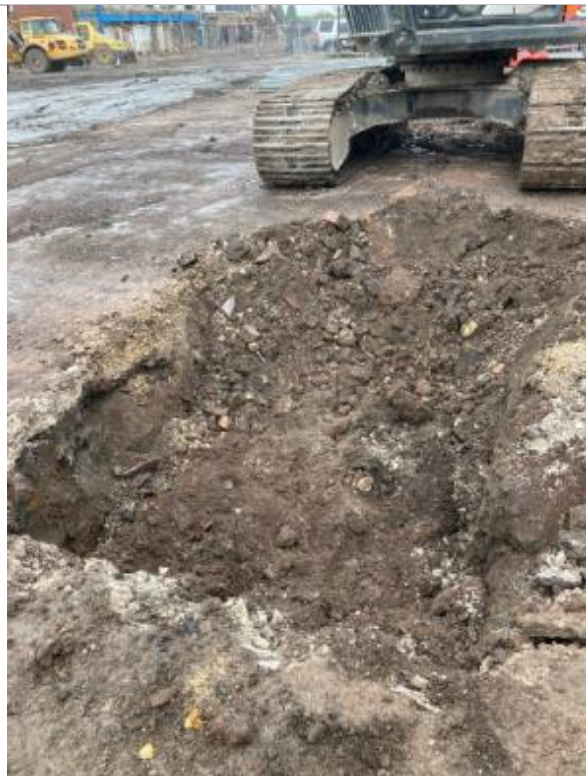
PLATE 16 ASBESTOS HOTSPOT TP303
