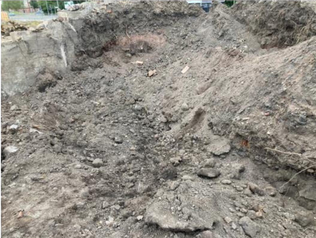
PLATE 17 ASBESTOS HOTSPOT- TP408 WITH VISIBLE ACM
