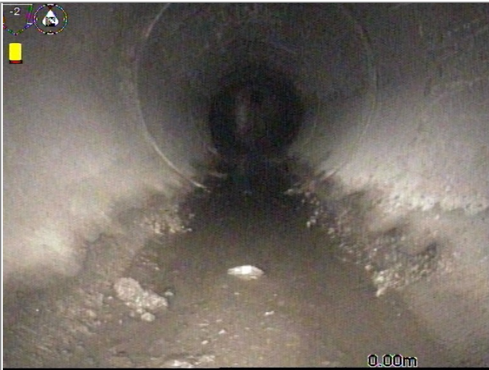
Start node type, manhole, reference S46
