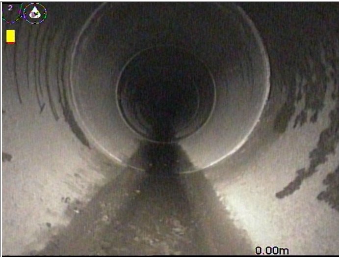
Start node type, manhole, reference S46
