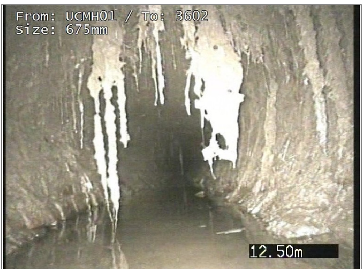
- Junction at 11 o'clock, diameter 150mm, Changed
