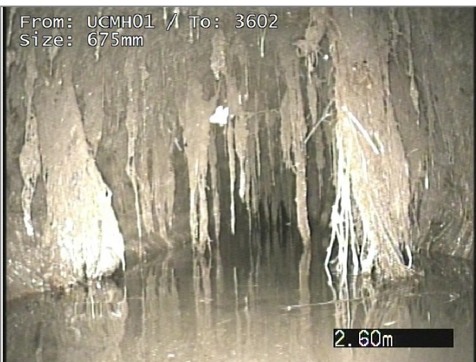
- Settled deposits fine 10% cross-sectional area loss, Changed
