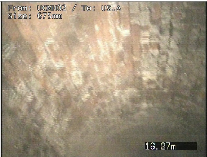
- Settled deposits fine 10% cross-sectional area loss, Changed
