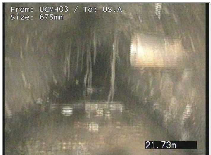
- Connection intruding at 3 o'clock, diameter 150mm, intrusion 15%, Changed
