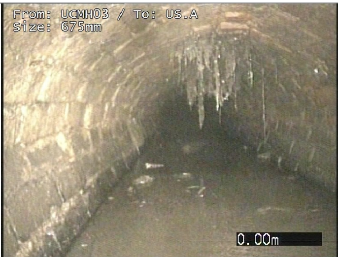
- Settled deposits fine 15% cross-sectional area loss, Changed
