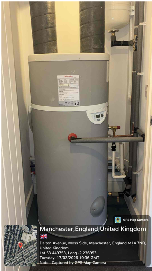
6A / 6B – plot 5 – ASHP and insulation to pipework
