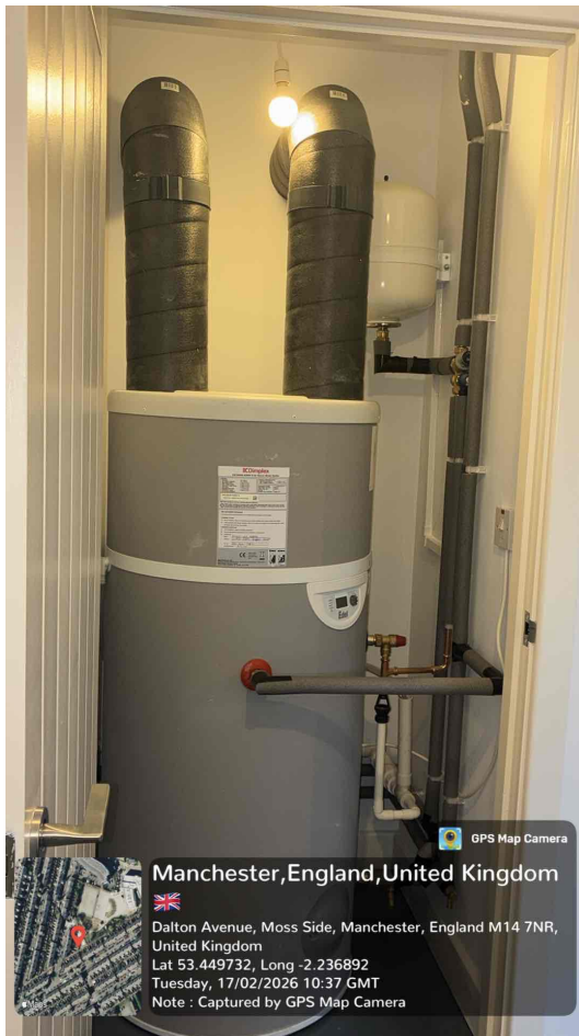
6A / 6B – plot 5 – ASHP and insulation to pipework
