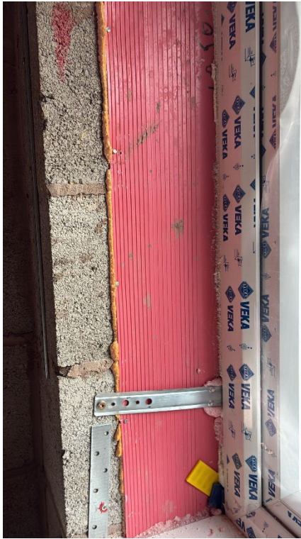
4A, 4B (E4) - plot 5 - window and thermabate junction
