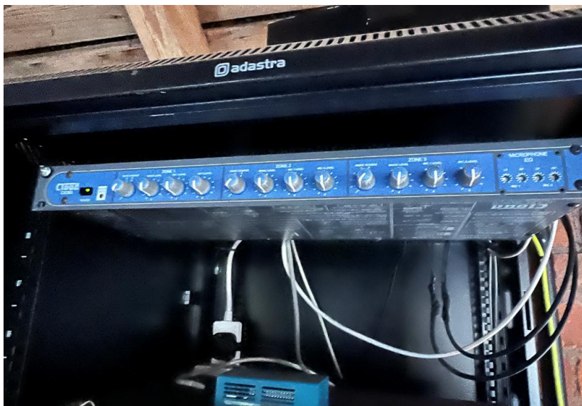
Figure 6 Photograph of volume controller unit (event space)
