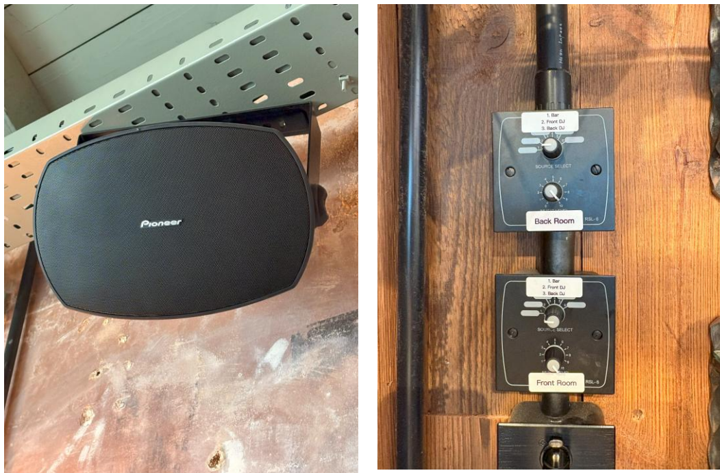
Figure 4 Photograph of loudspeaker and controller unit
