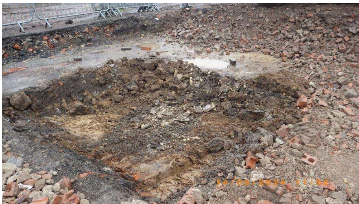
NT03 Northern area...asbestos cement materials encountered during excavations for site cabins (see Section 4.2). 14 th May 2024
