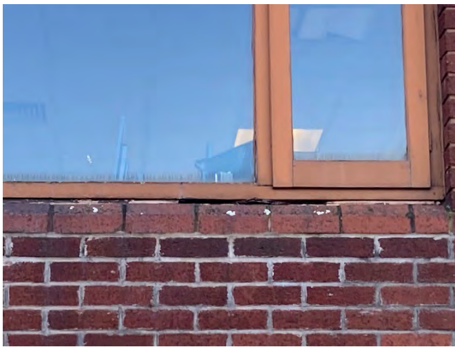
Photograph 17: Gaps in mortar surrounding windows on level 5 flat roof
