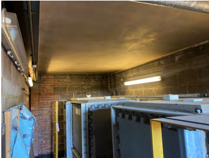
Photograph 16: 6 th floor tank room
