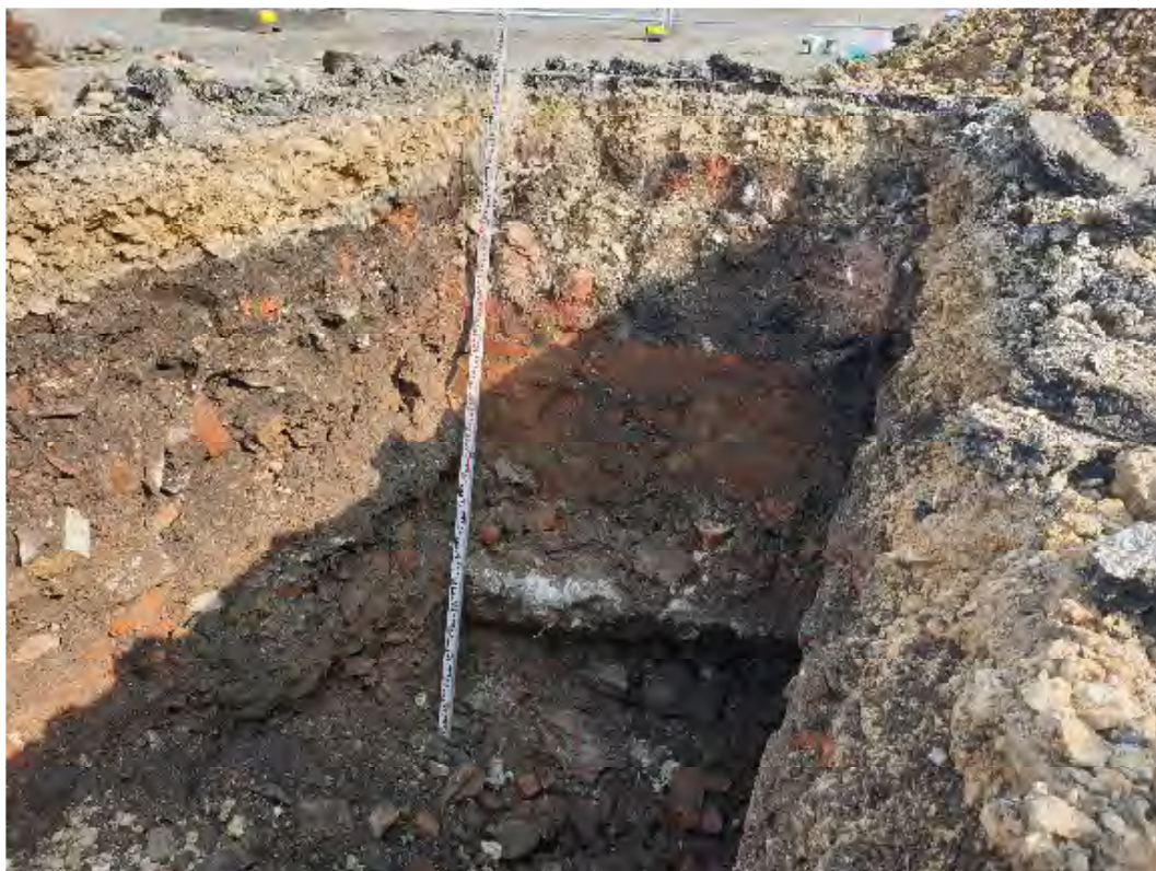
Photo No. 6: TPI03
