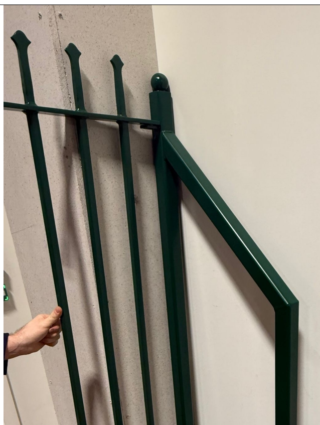
Sample panel of fencing and cracked posts as inspected on site
