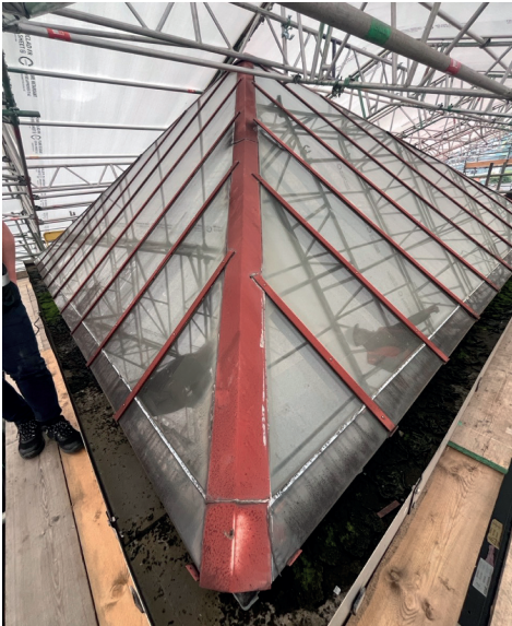
Image 14: Existing rooflight in poor condition glazing bars and glass.
