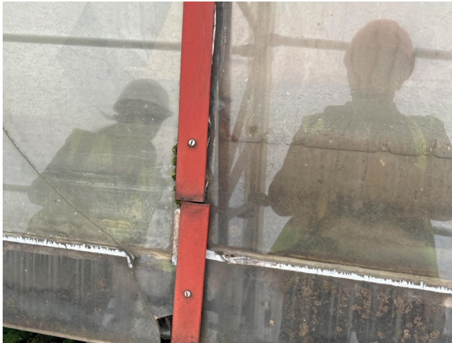
Image 191: Detailed view of existing failing lantern light.
