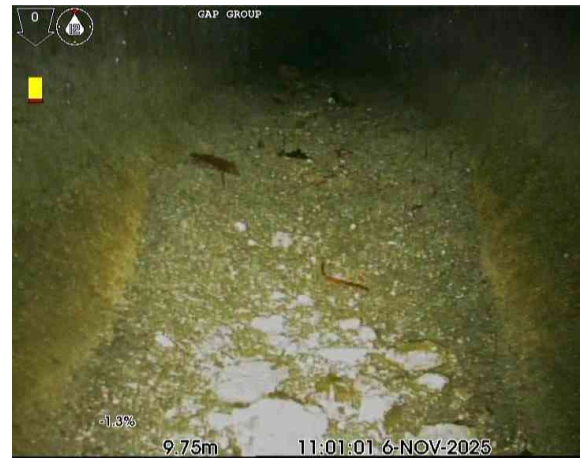
2, 00:01:08, 9.75 m Settled deposits, fine, 15% cross-sectional area loss, start
