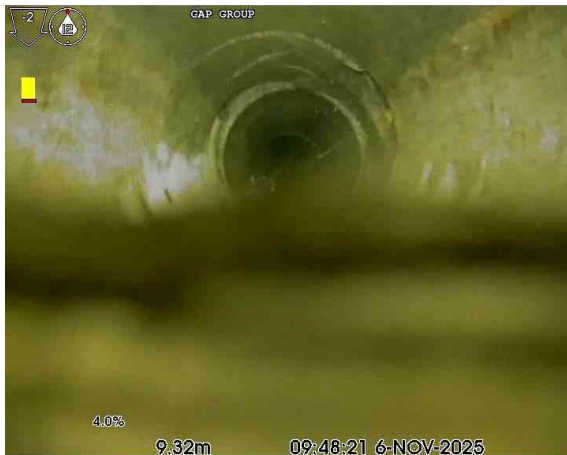
1, 00:01:35, 9.85 m Cracks, multiple from 12 o'clock to 12 o'clock
