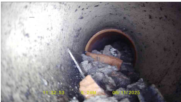
3, 00:00:50, 5.24 m Other obstacles, brick or masonry in invert at 6 o'clock, 100% cross-sectional area loss
