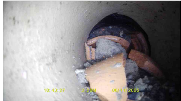
2, 00:00:21, 3.26 m Collapsed drain or sewer, 100% cross-sectional area loss
