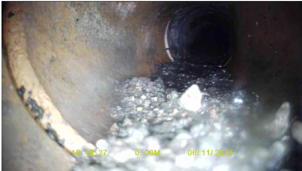
1, 00:00:05, 0.00 m Settled deposits, fine, 10% cross-sectional area loss, start
