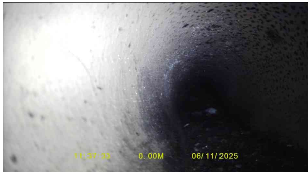
1, 00:00:05, 0.00 m Settled deposits, fine, 20% cross-sectional area loss, start
