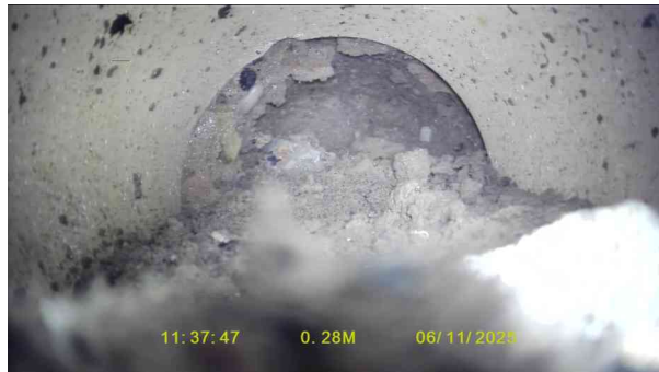
2, 00:00:19, 0.28 m Settled deposits, fine, 100% cross-sectional area loss
