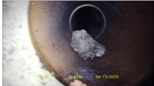
2, 00:00:10, 0.97 m Other obstacles, brick or masonry in invert at 6 o'clock, 30% cross-sectional area loss
