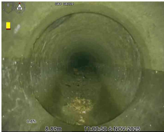
1, 00:00:57, 8.89 m Joint displaced, large
