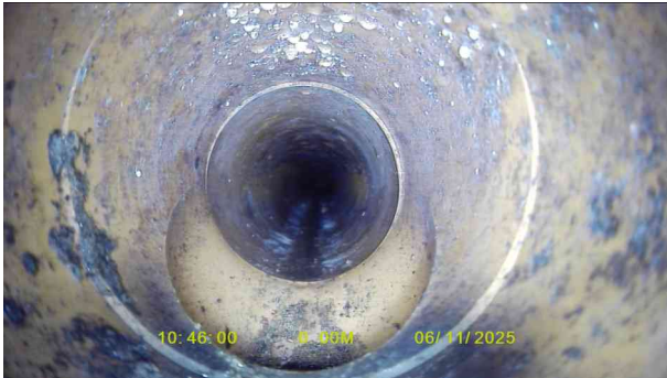
1, 00:00:05, 0.10 m Junction at 6 o'clock, 100mm dia, BACKDROP
