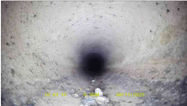
1, 00:00:04, 0.00 m Settled deposits, fine, 5% cross-sectional area loss, start
