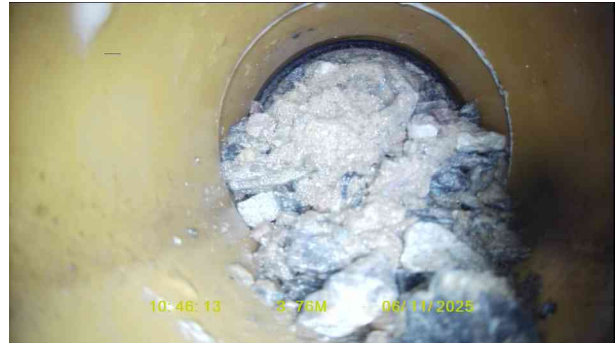
2, 00:00:18, 3.76 m Settled deposits, hard or compacted, 100% cross-sectional area loss, STONES
