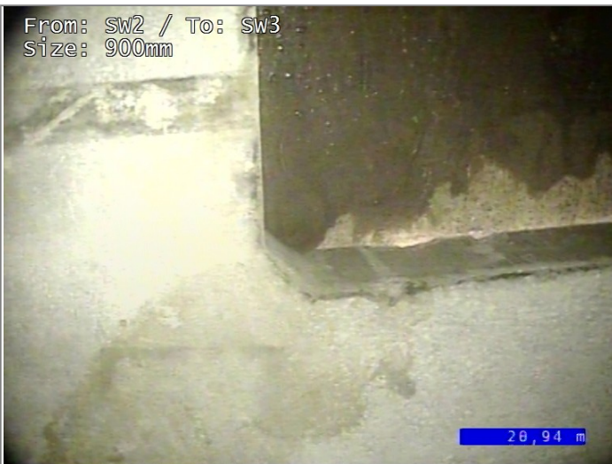
Finish node type, manhole, reference SW3
