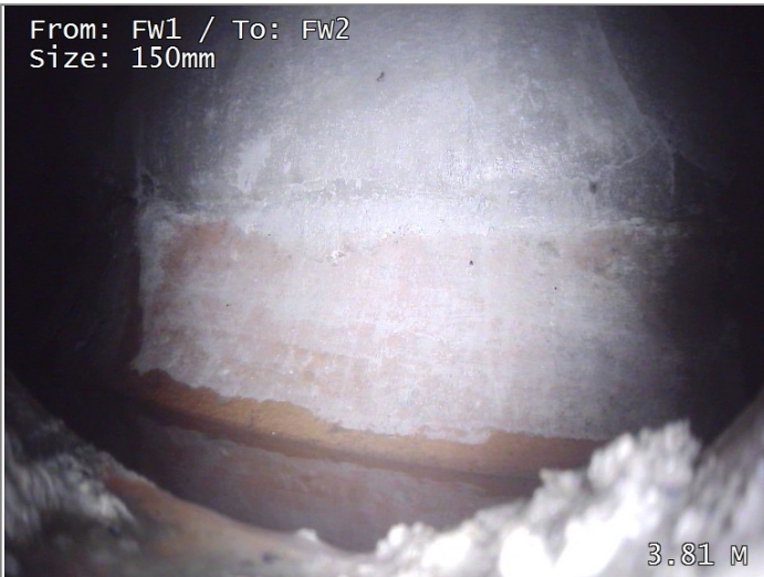
Finish node type, manhole, reference FW2
