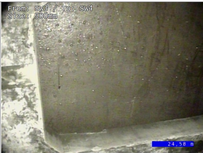
Finish node type, manhole, reference SW4
