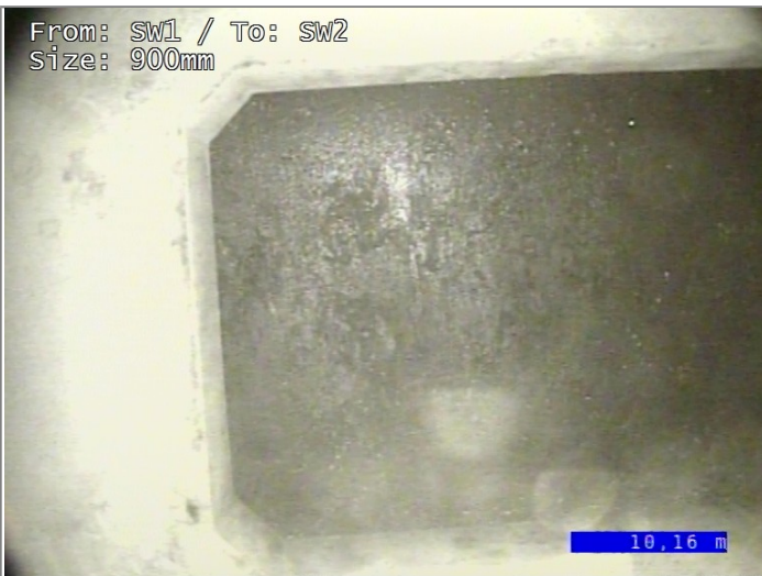
Finish node type, manhole, reference SW2
