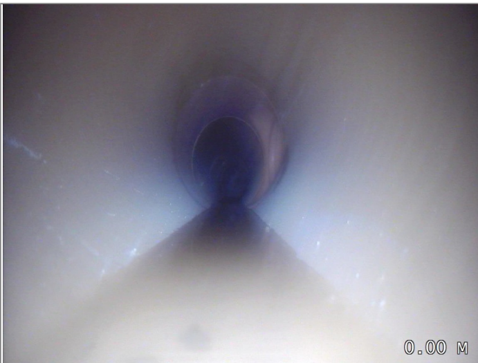
Start node type, manhole, reference SW1
