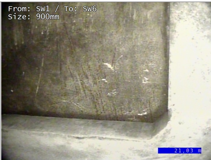
Finish node type, manhole, reference SW6
