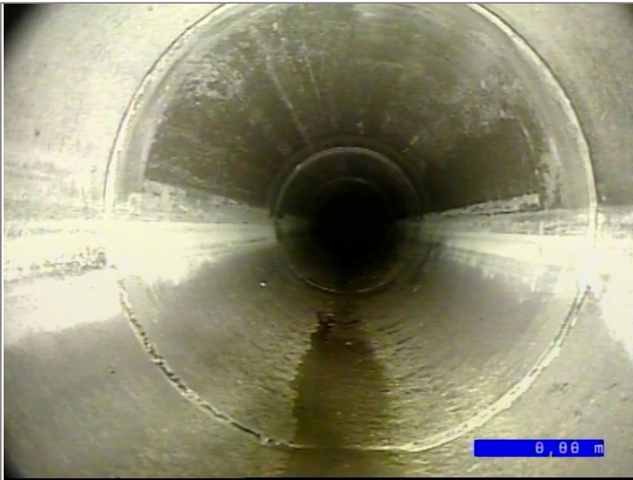
Start node type, manhole, reference SW1
