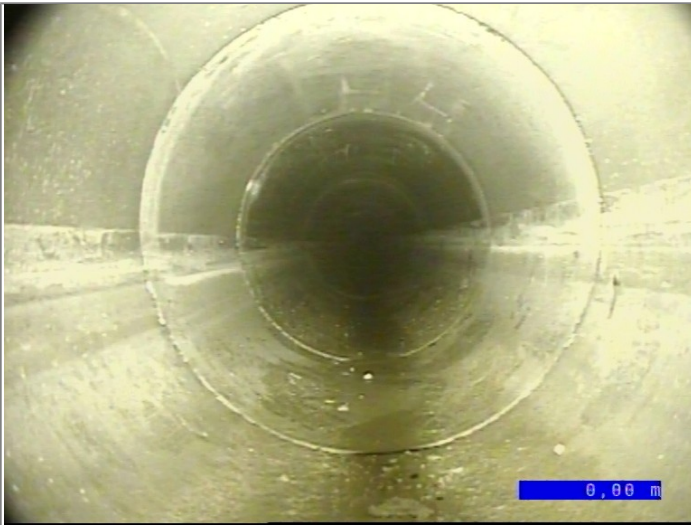
Start node type, manhole, reference SW2
