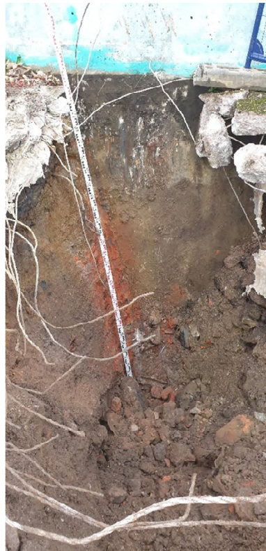
Plate No.14: PP TP109 – foundation of retaining wall not found due to depth and pit instability
