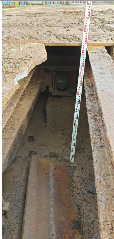
Plate No.22: PP TPI12 – Weighbridge - internal
