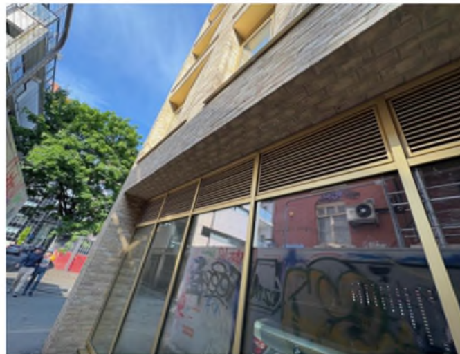
Previously approved louvres in situ on Block B
