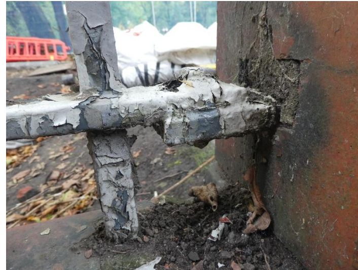
Figure 10: evidence of underlying darker grey paint finish
