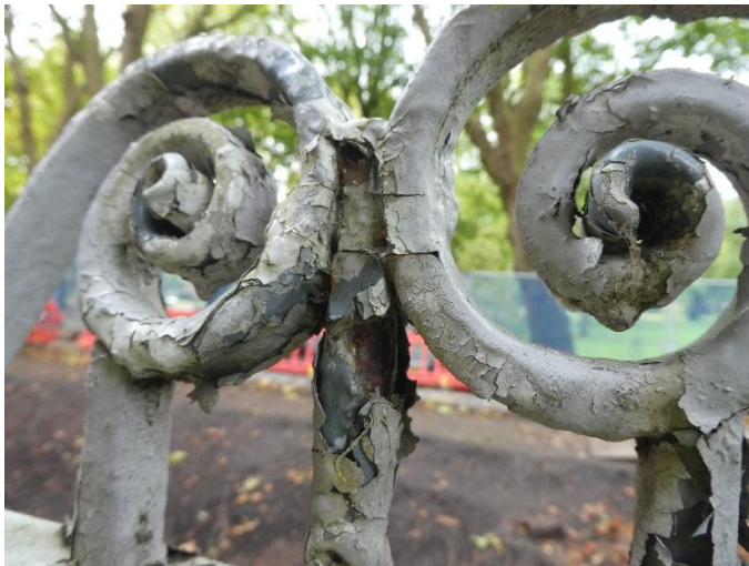
Figure 9: example of the poor condition of the paint finish to the railings as seen during site survey
