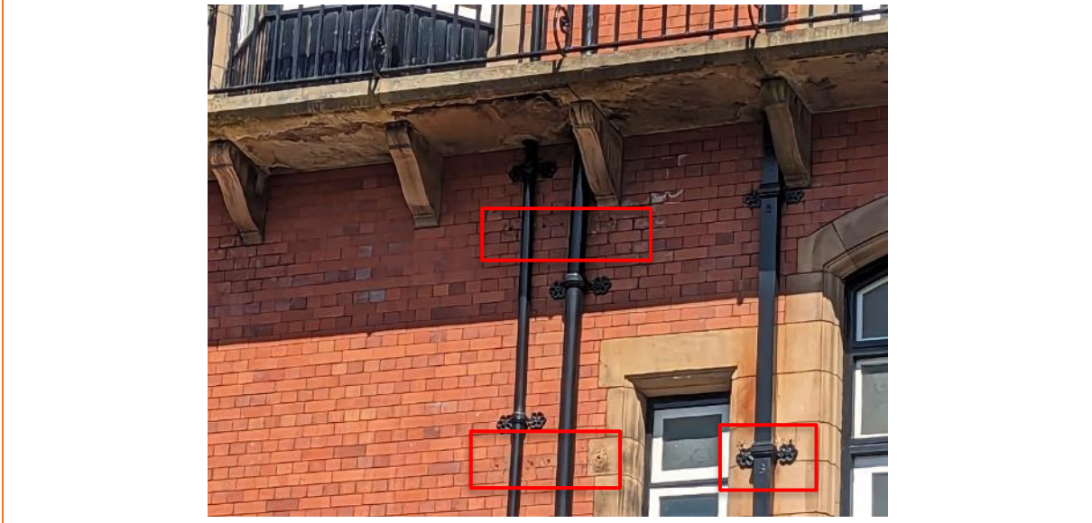
PLATE 2 SHOWING SMALL HOLES IN THE BRICKWORK AND STONE
