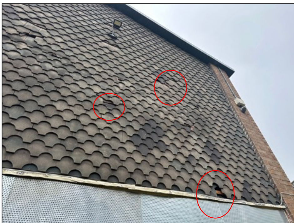
Photograph 7; A front view of the clay tile cladding exterior. Again, damage was noted and lead directly to the external wall, with crawlspace between the tiles and the wall. This cladding sits atop the external wall and does not lead to the internal composition.
