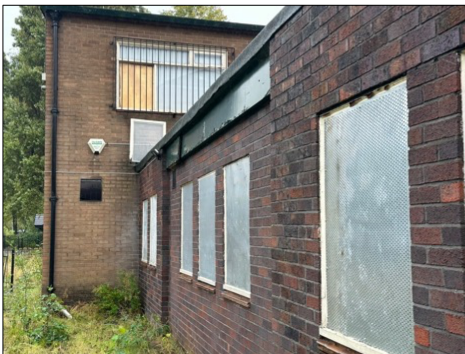
Photograph 4; A view of the front of the subject building, beneath one of the single storey, flat roof sections. External fascia boarding shows some sign of rotting and cosmetic damage. External windows are boarded.
