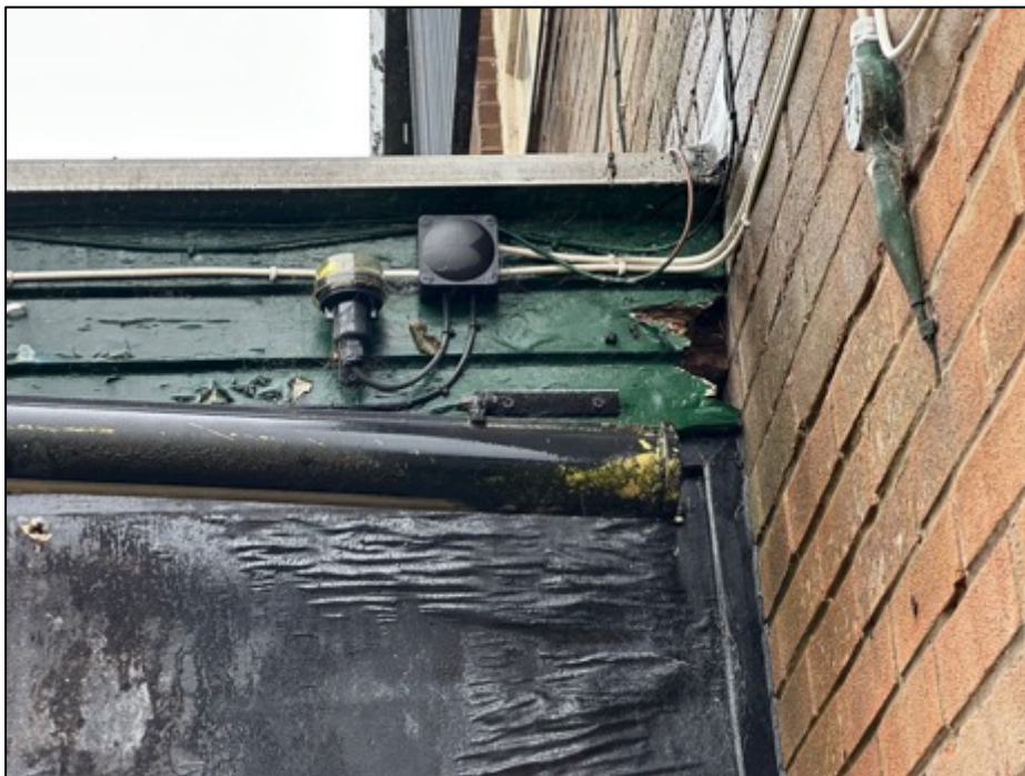
Photograph 10; A view of further fascia boarding which shows signs of damage, notably at an intersection of the single storey section with the larger building.
