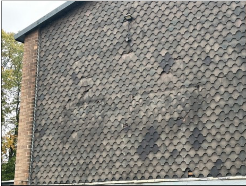
Photograph 5; Clay cladding tiles feature on the front face, with some instances of damage noted.
