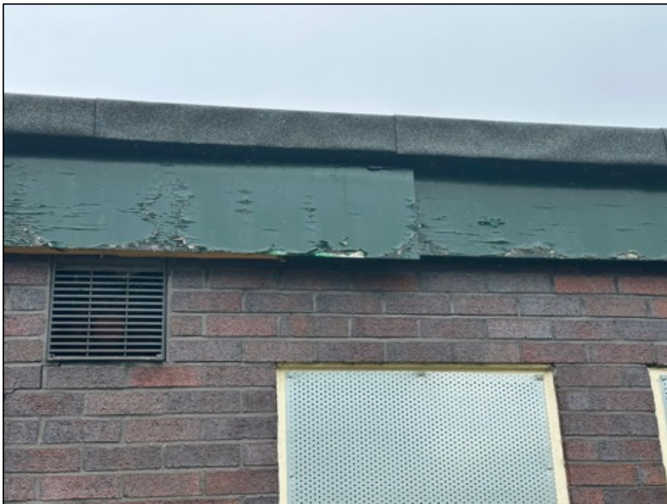
Photograph 6; A view of some wooden fascia boarding, which is detached from the external walls and damaged. This paneling is set away from the wall, and when investigated does not lead to internal cavity space or roof space.
