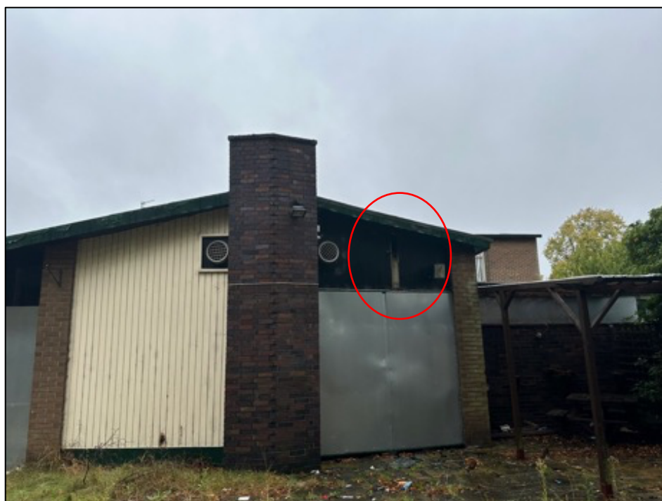
Photograph 8; A view of the northeastern face of the building, where the former outdoor seating area was located. The single storey section features damage to external wooden wall panels (circled).
