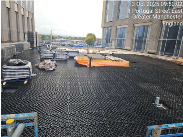
Block 3 Blue Roof Attenuation Crates Photo
