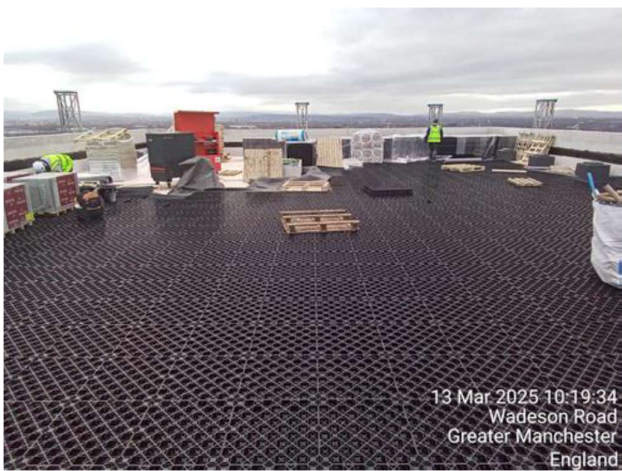
Block 2 Blue Roof Attenuation Crates Photo
