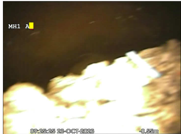
Photo: 10_4b, 00:00:00 0.1m, Debris, 20 % cross-sectional area loss
