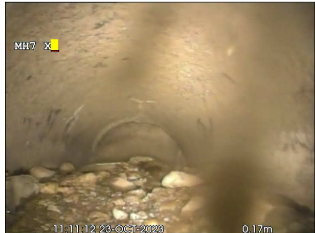
Photo: 104_5a, 00:00:00 0.3m, Debris silt, 10 % cross-sectional area loss, Start
