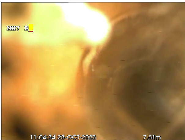
Photo: 97_6a, 00:00:00 7.6m, Dimension of sewer changes, new dimension dia 100 mm
