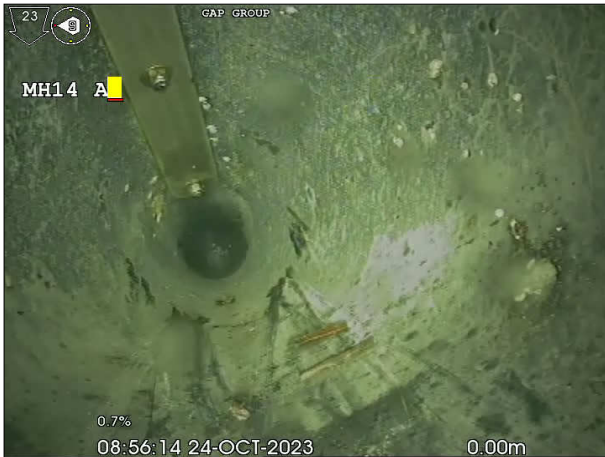
Photo: 214_4a, 00:00:00 0.1m, General Observation, Remark: Sewer reappear
