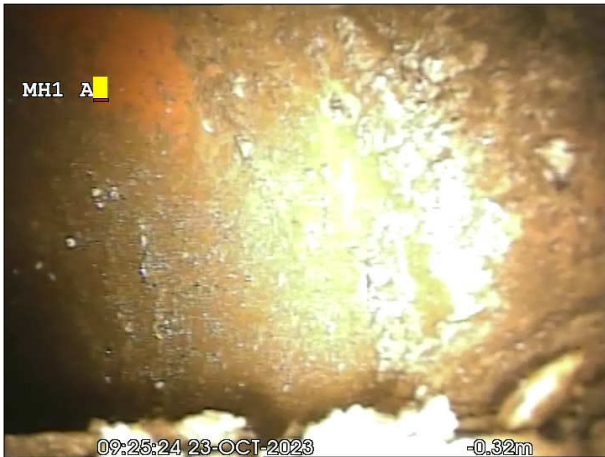
Photo: 10_4a, 00:00:00 0.1m, Debris, 20 % cross-sectional area loss
