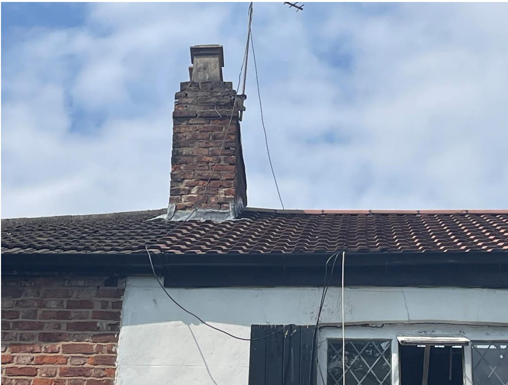
PHOTO 5 – LEANING CHIMNEY STACK
