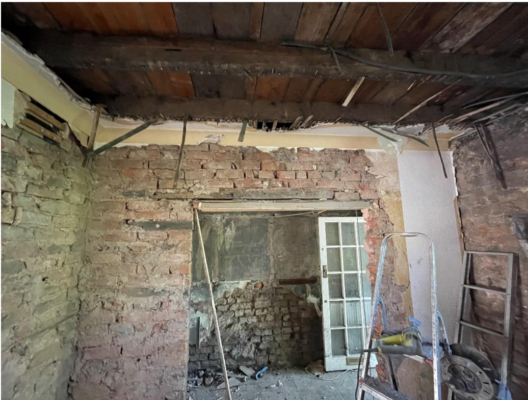
PHOTO 13 – UNSUPPORTED INTERNAL TIMBER LINTEL BEAM
