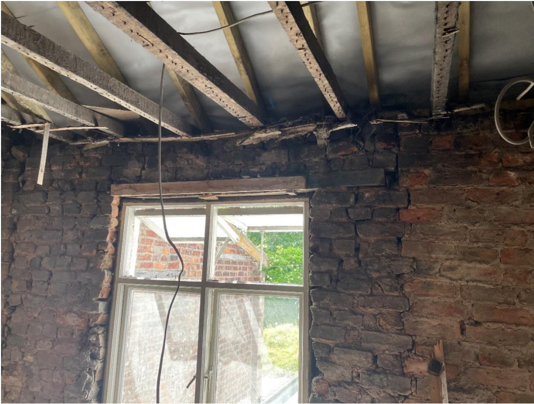
PHOTO 9 – LOCALLY CRACKED AND DISPLACED BRICKWORK AT LINTEL BEAM BEARING
