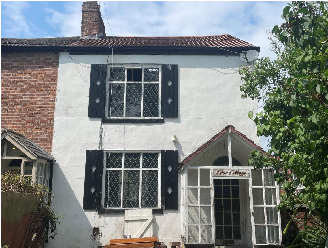
PHOTO 1 – FRONT ELEVATION – UNEVEN ROOF STRUCTURE
