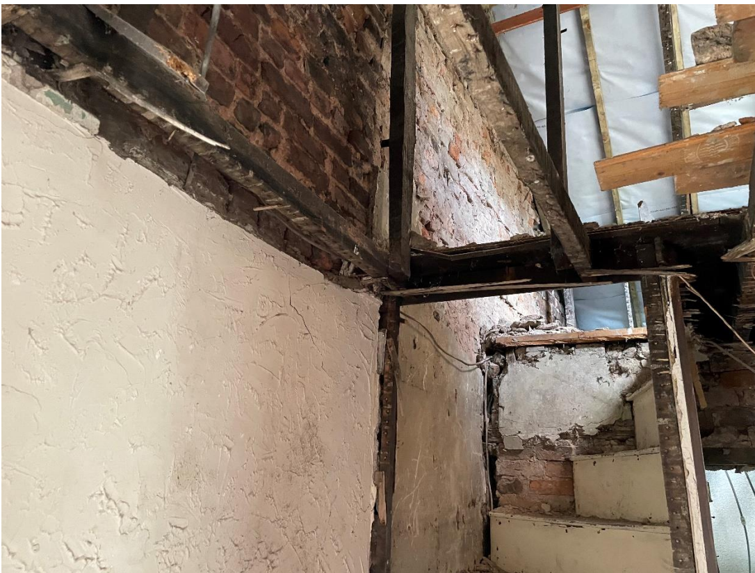
PHOTOS 7 & 8 – VERTICAL SEPARATION CRACKS IN BRICKWORK
