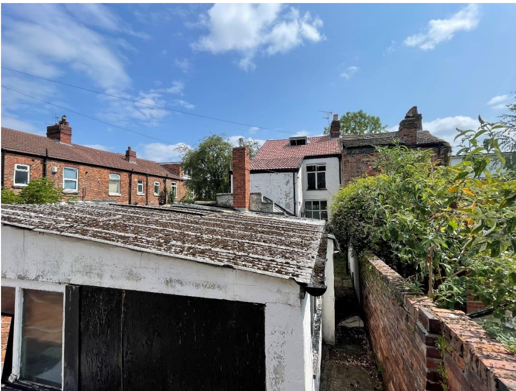
PHOTO 6 – PERISHED ROOF COVERINGS OVER SINGLE STOREY REAR EXTENSIONS
