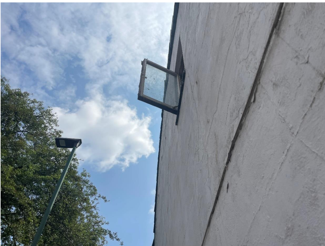
PHOTOS 3 & 4 – BADLY DEFLECTED GABLE WALL
