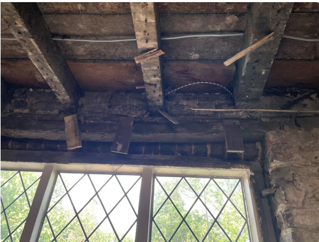
PHOTO 12 – INADEQUATE TIMBER LINTEL BEAM
