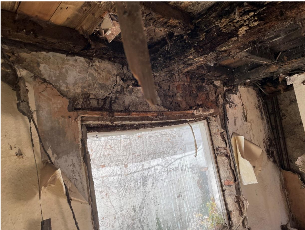
PHOTO 10 – ROT INFECTED TIMBER FLOOR BEAM AND LINTEL
