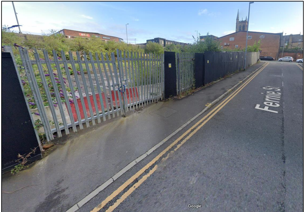
Figure 3-2 – Fernie Street – disused vehicular and pedestrian access gates
