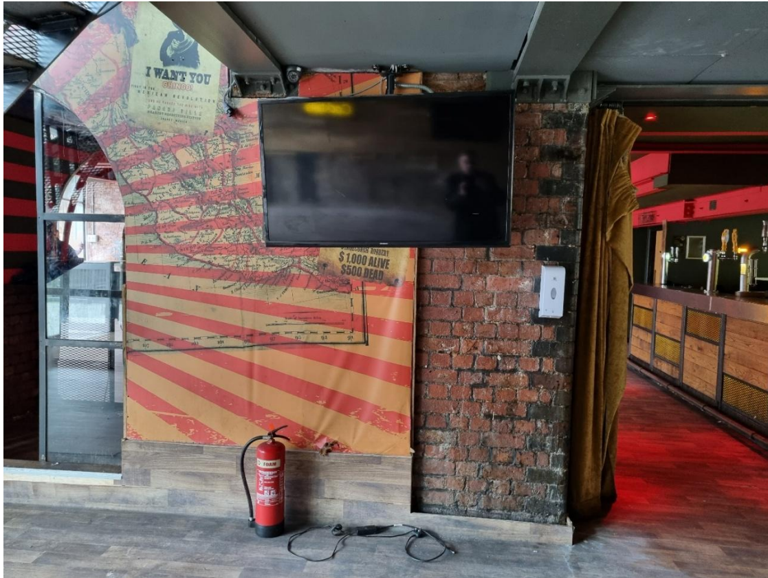
Water ingress to walls causing damage to tenant's fitout
