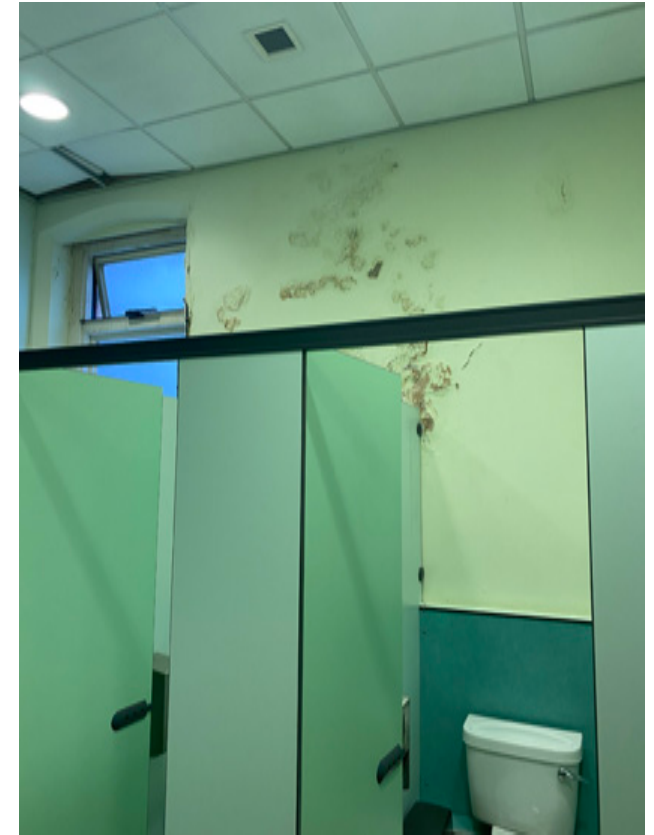
3.4.63 Room 2.055, women's WC, partition extending into 2.054
