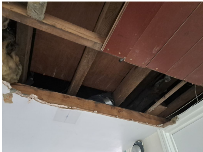
Internal damp damage from previous roof leaks
