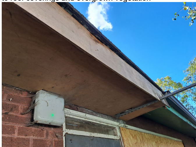
Defective and missing rainwater goods
