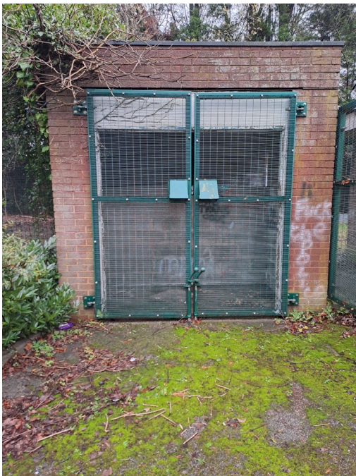
Bin store with defective steel lintel damaging and lifting brickwork
