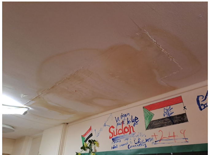
Internal damp damage and graffiti from previous squatters
