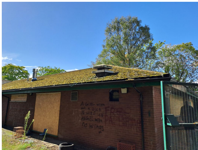
Rear elevation with graffiti to elevations
