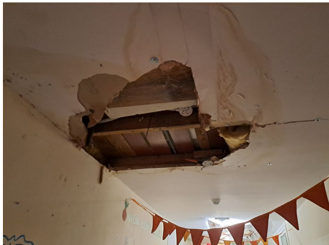
Internal damp damage from previous roof leaks
