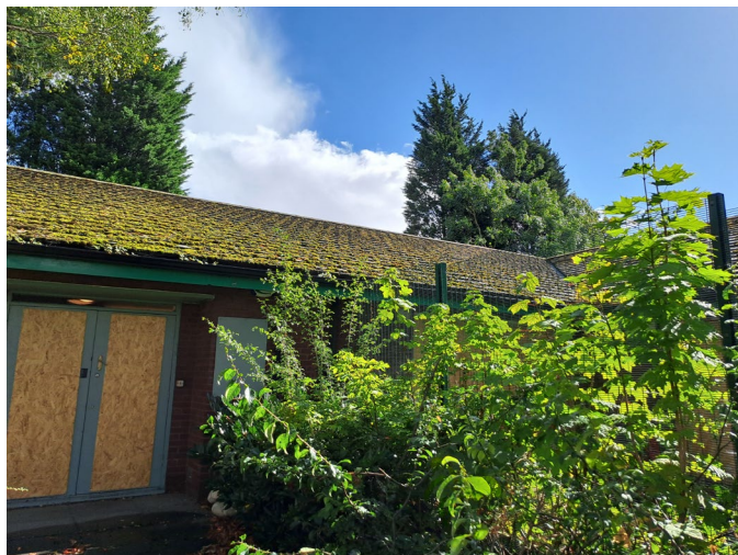
Front elevation with boarded up windows, moss growth to roof coverings and overgrown vegetation
