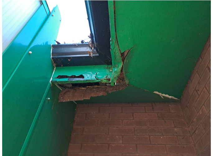
Defective rainwater goods and rotten timber eaves
