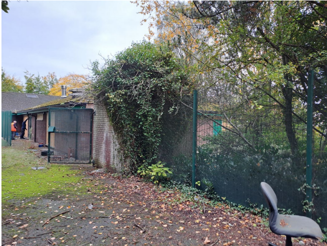
Overgrown vegetation to rear elevation of bin store
