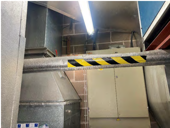
Photograph 14: Interior of 7 th floor plant room
