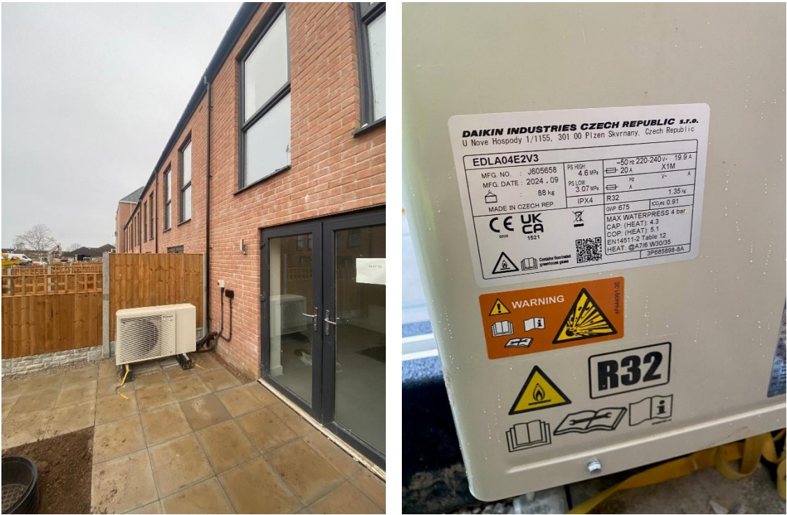
Photographs of typical heat pump install & model specification
