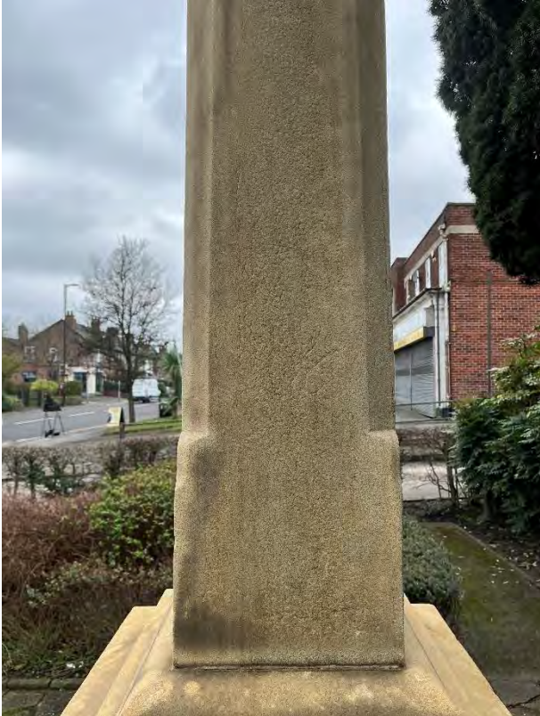
Photo 14 The layers of the stone are visible, there are in a vertical orientation. • Minor cracking/opening up of minor fissures (too aggressive cleaning or natural weathering?)
