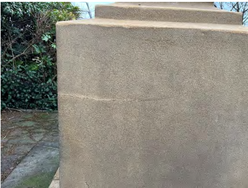
Photo 18 Horizontal crack 2/3 way up left side, running from rear edge for ½ width
