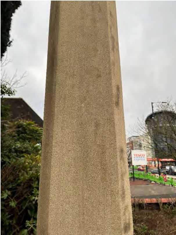
Photo 11 The layers of the stone are visible, there are in a vertical orientation. 2 very minor areas of iron staining (horizontal - 30-40mm long x 0.5mm, with very mild rust staining running down the surface)
