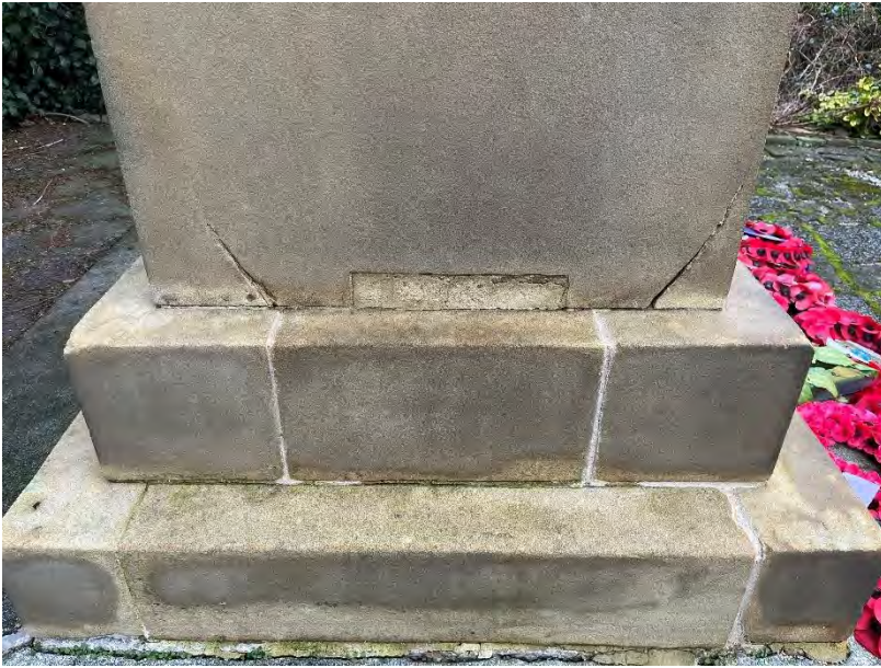
Photo 19 Failing, poor quality repair on bottom edge. 2 diagonal cracks on bottom corners
