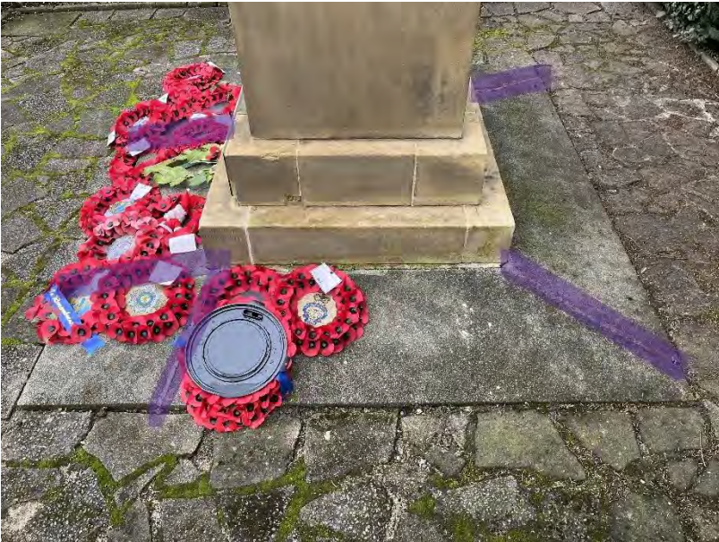
Photo 46 right side of apron showing cracks (highlighted in purple)
