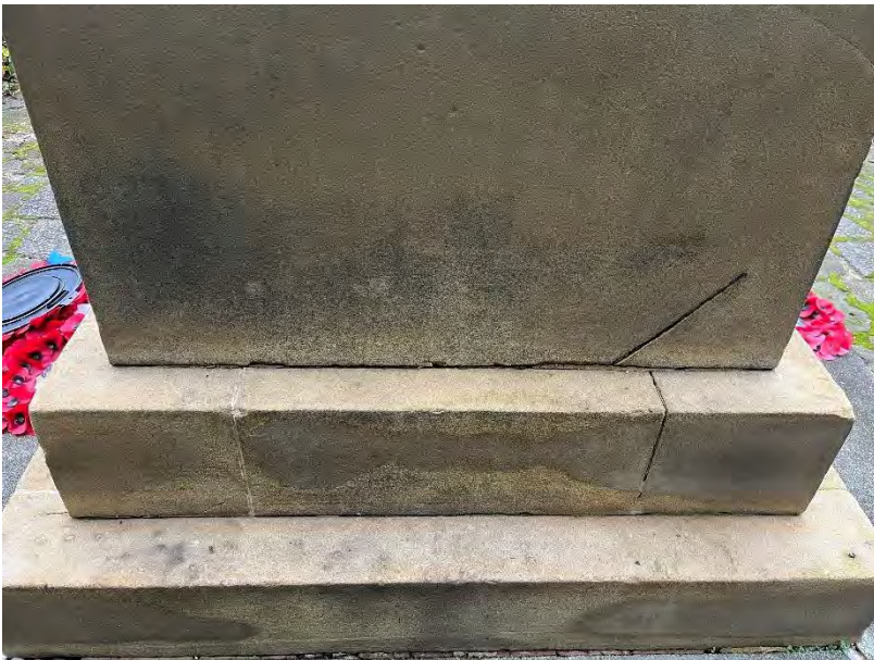
Photo 22 Bottom edge damaged
