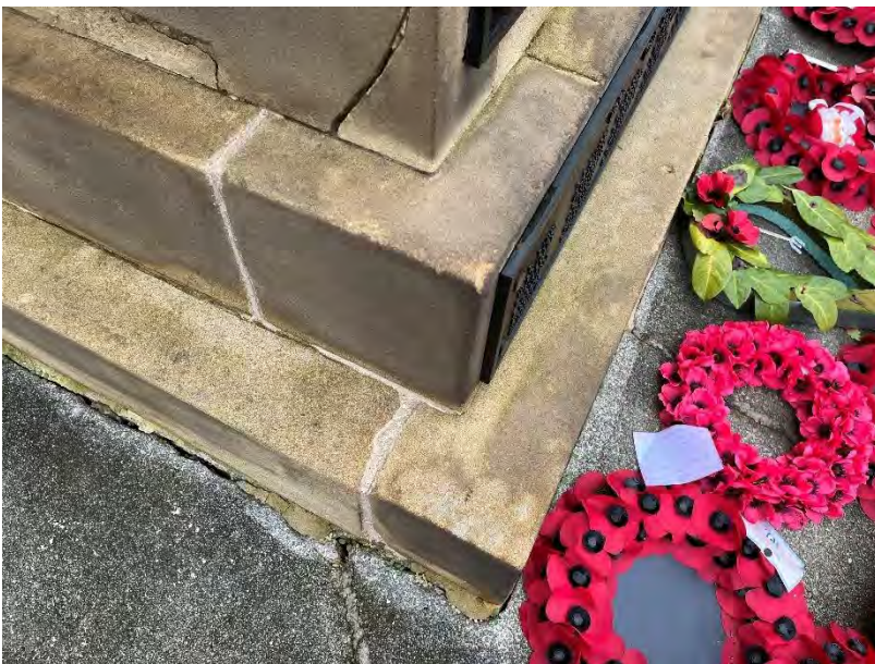
Photo 26 minor damage to top front corner
