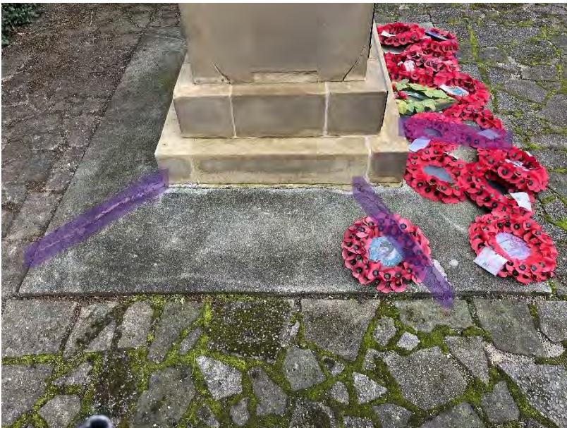
Photo 44 left side of apron showing cracks (highlighted in purple)
