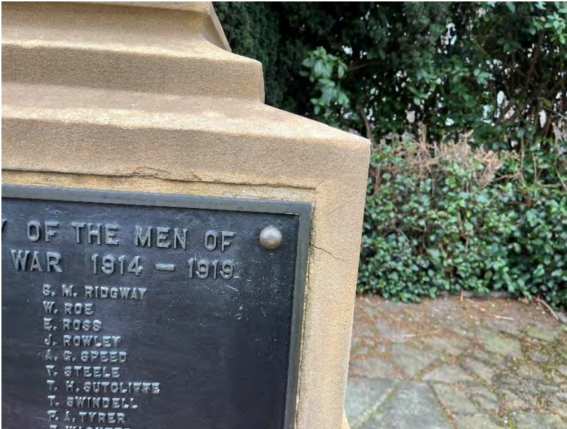
Photo 17 crack across bolt in upper right corner of plaque
