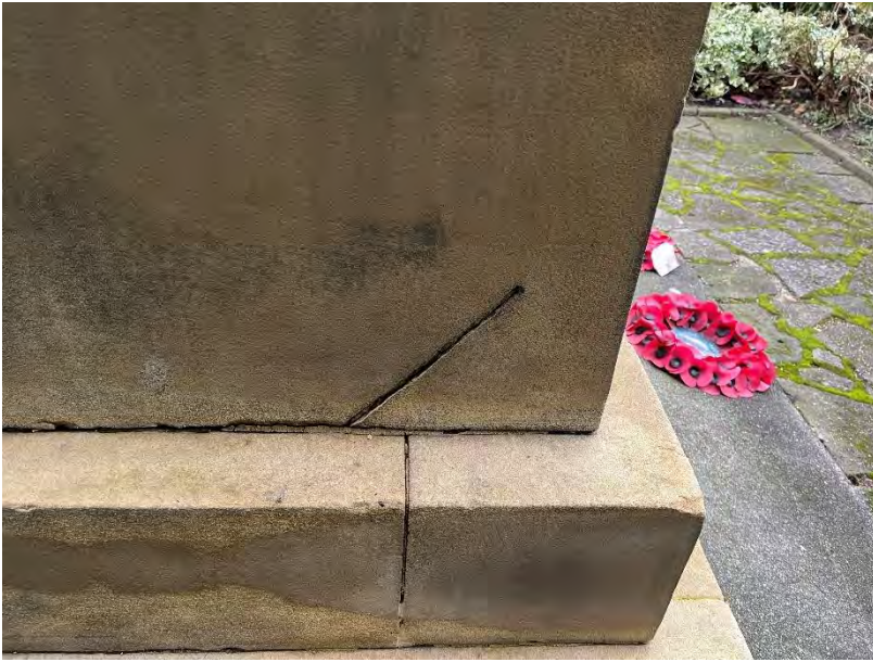
Photo 21 Diagonal crack to lower left corner
