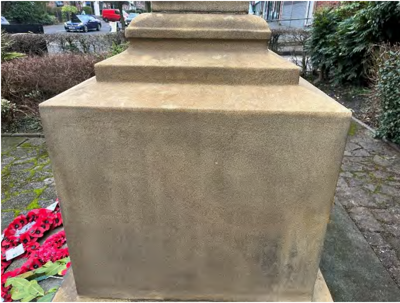
Photo 23 Minor pitting to upper vertical surface, upper surface – very aggressively cleaned by pressure washer, slight damage to original smooth surface
