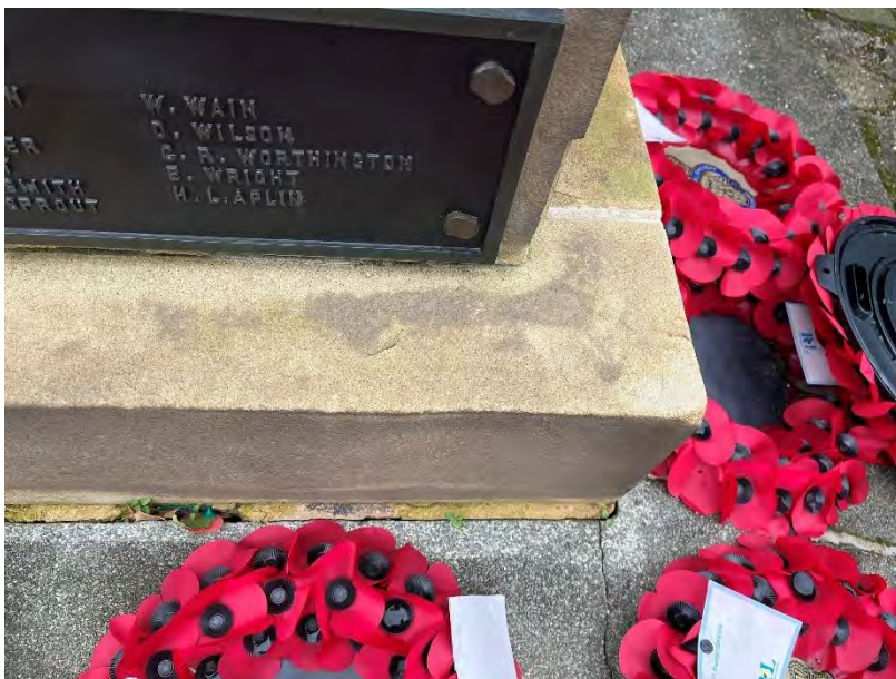
Photo 36 minor area of damage to the upper surface at RHS
