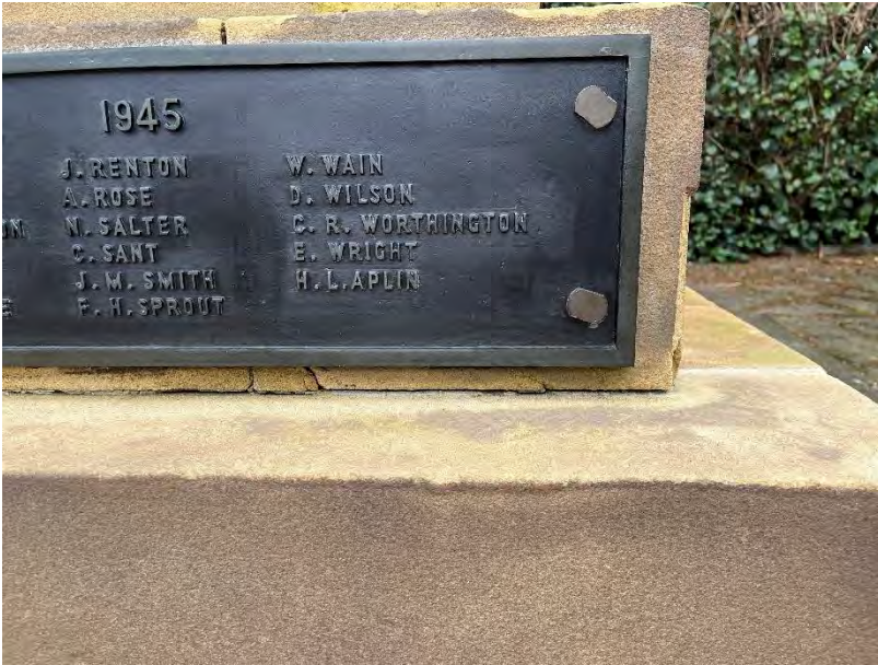
Photo 25 Right hand block diagonal crack below plaque, LHS of block Left
