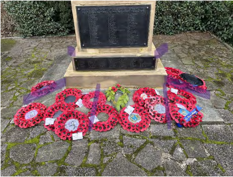
Photo 43 front apron showing cracks (highlighted in purple)
