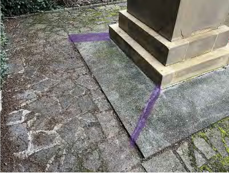
Photo 45 rear of apron showing cracks (highlighted in purple)
