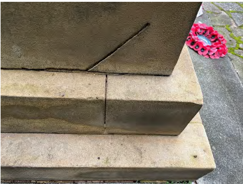
Photo 30 joint between left rear corner stone and rear intermediate stone open-jointed
