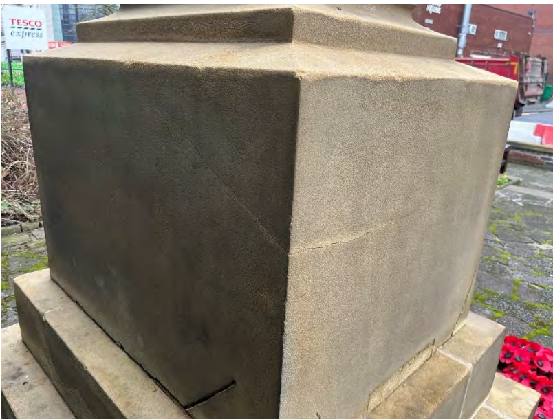
Photo 20 Continuation of horizontal crack (see Photo 18), but heading diagonally up
