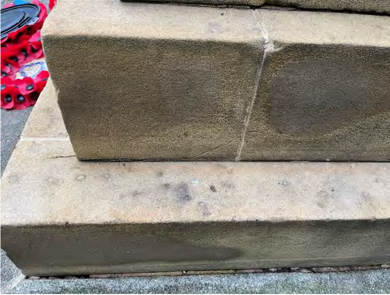
Photo 31 Right block, small diagonal crack
