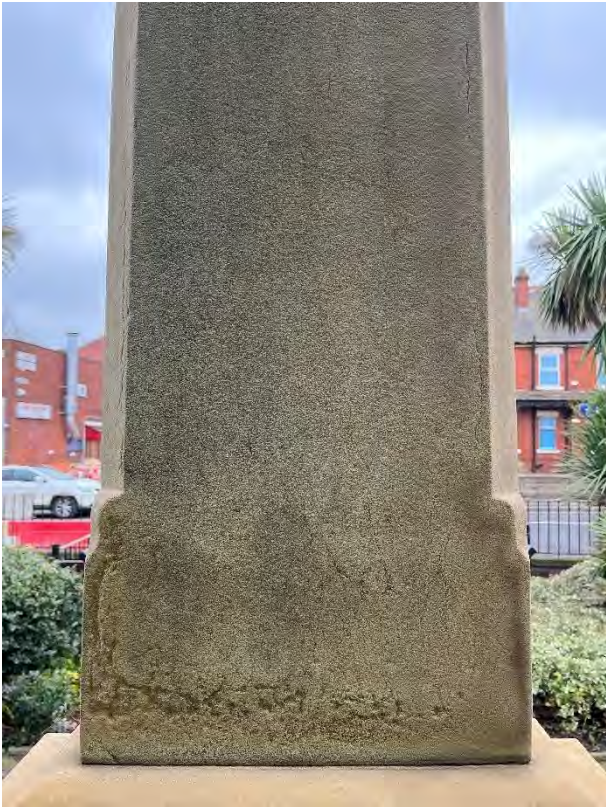
Photo 13 Minor pitting/spalling of stone at bottom of shaft (too aggressive cleaning or natural weathering?)
