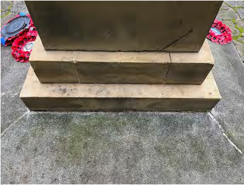
Photo 39 some staining on upper surface
