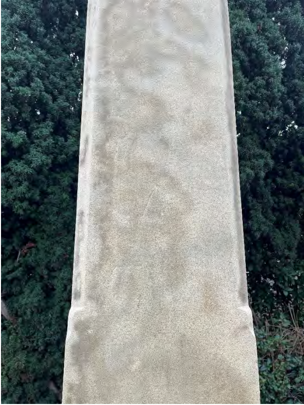
Photo 10 shaft - front elevation showing minor weathering to surface/possible too aggressive cleaning
