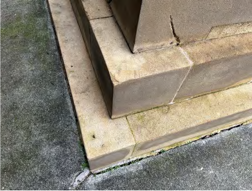
Photo 27 damage to top rear corner
