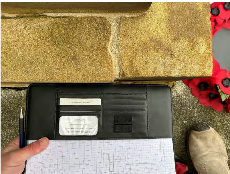
Photo 38 The middle stone has been displaced to the left
