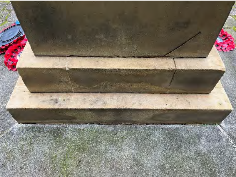
Photo 32 Slight spalling/aggressive cleaning
