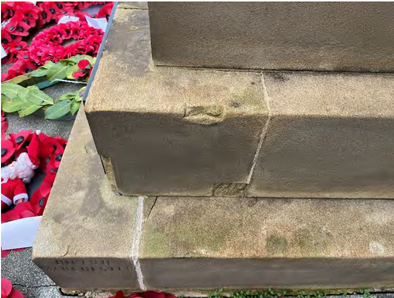
Photo 34 Front block has 2 damaged areas with corner damage (as noted on Photo 24)
