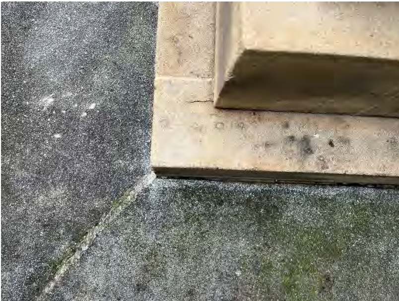
Photo 40 minor crack on upper surface to RHS
