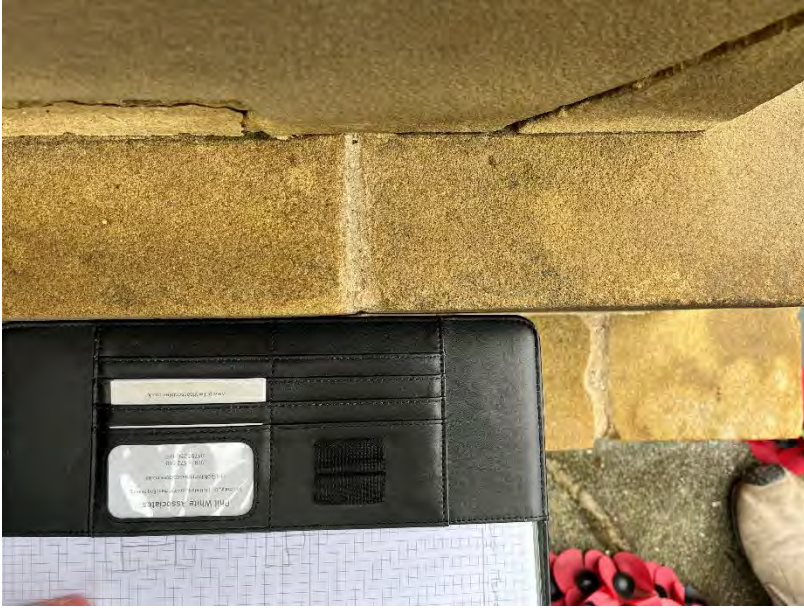
Photo 29 Misalignment between middle and front block
