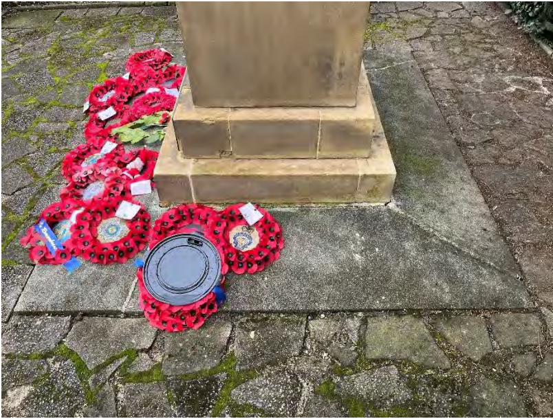
Photo 41 both vertical joints have been repointed, both joints are wide, especially the forward vertical joint
