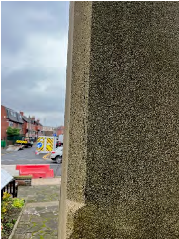
Photo 12 Very minor cracking parallel to the vertical vertices of the chamfers
