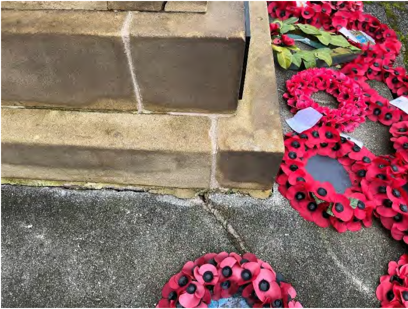
Photo 37 Very wide front joint between front and side stones, which has been repointed
