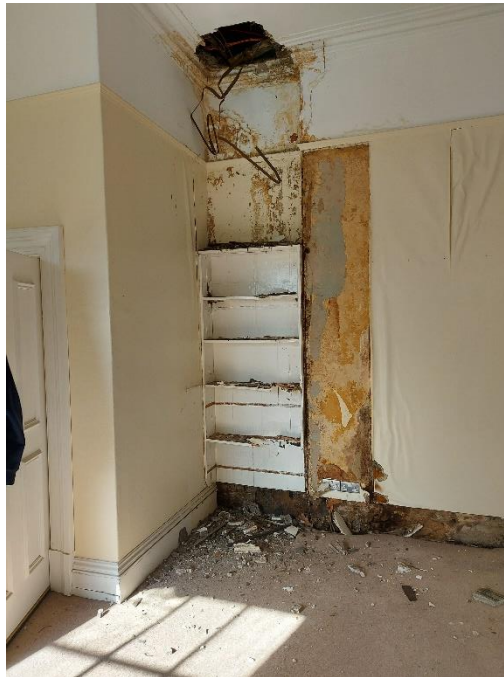
Photograph 1 Room 1.107 – rafter feet exposed
