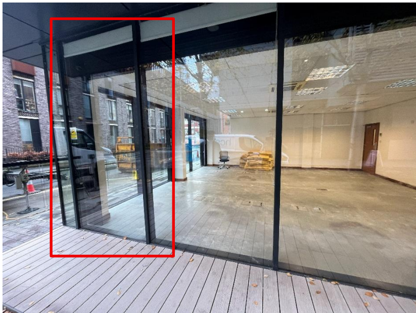
Glazed window to be replaced with door on Burton Place
