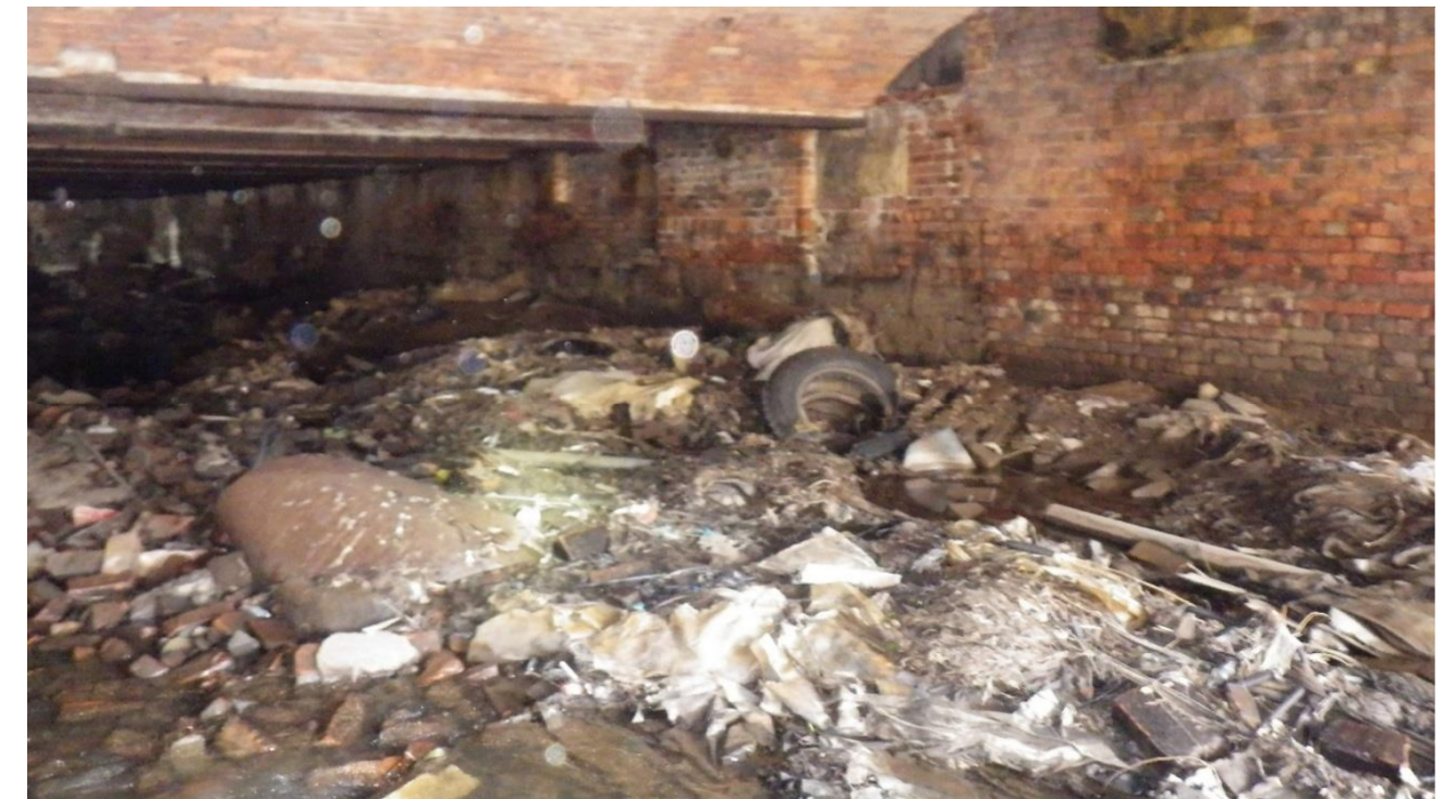
Figure 5-3 Debris build up within culvert
