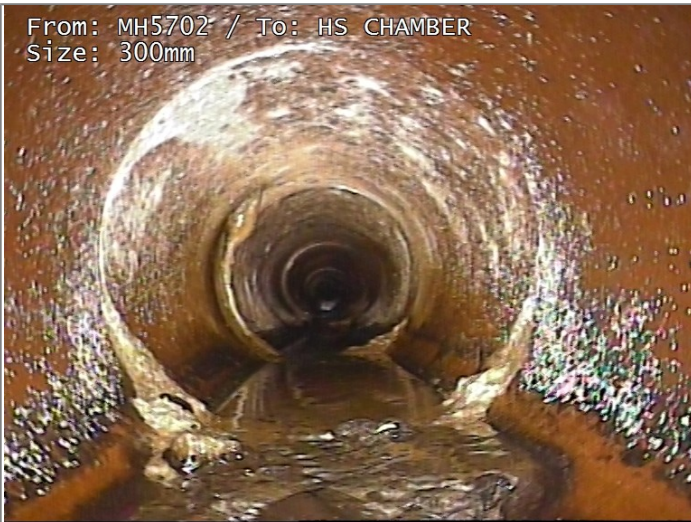
Settled deposits hard or compacted 10% cross-sectional area loss
