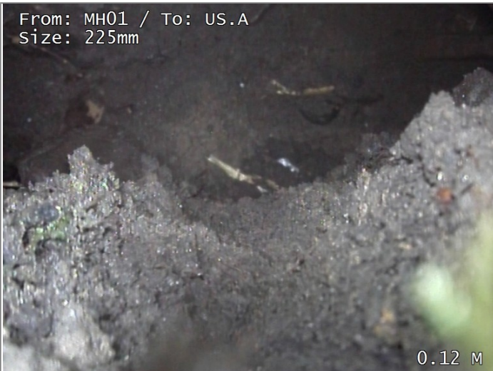
Settled deposits fine 70% cross-sectional area loss
