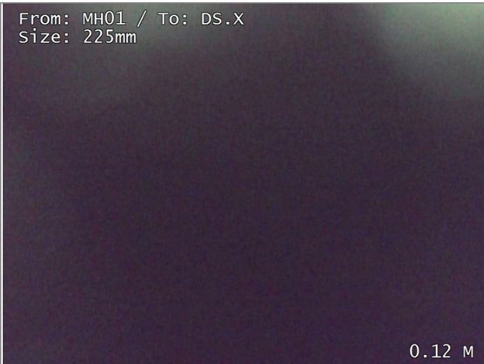
Settled deposits fine 90% cross-sectional area loss
