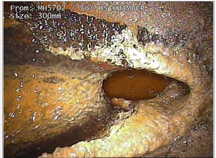
Junction at 11 o'clock, diameter 100mm - Remark: ENCRUSTATION AROUND JUNCTION
