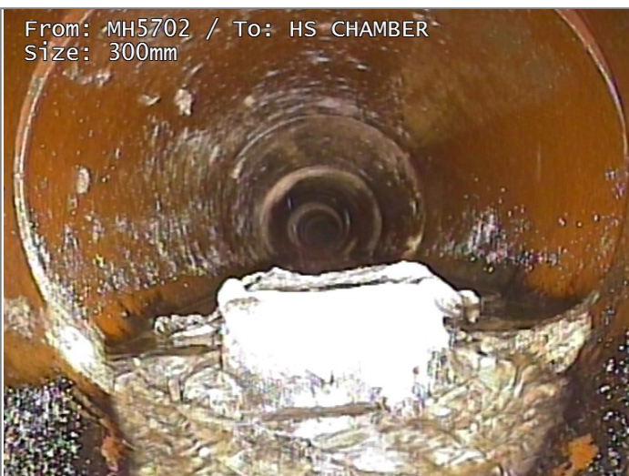
Settled deposits hard or compacted 30% cross-sectional area loss
