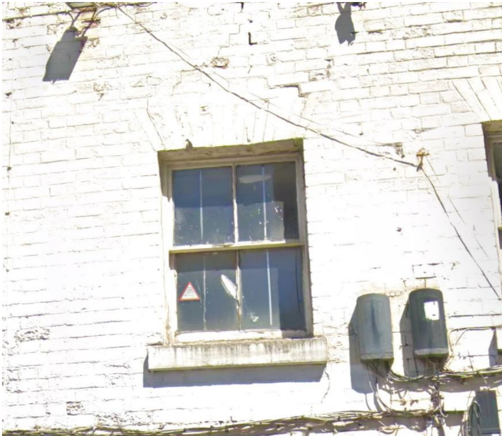
Photo showing failed lintel and diagonal triangular cracking above window
