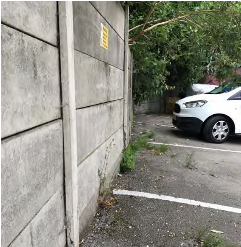
3. Bulging and cracking of retaining wall.
