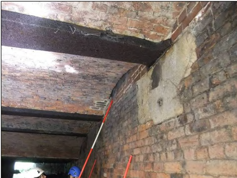
Plate 4 Culvert B24 showing gaps at junction between wall and roof
