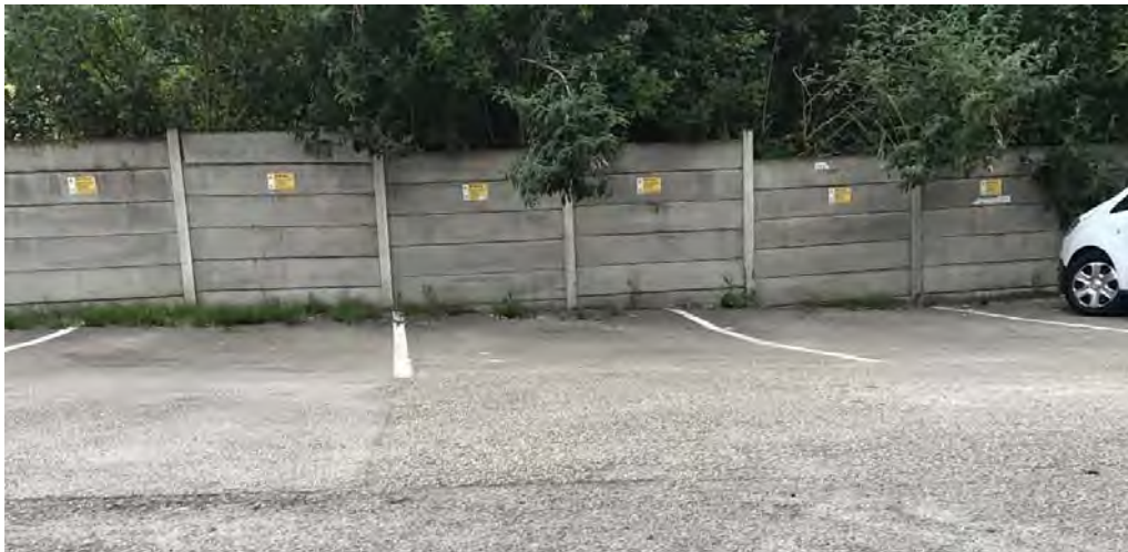
4. Depression in tarmac in front of retaining wall.
