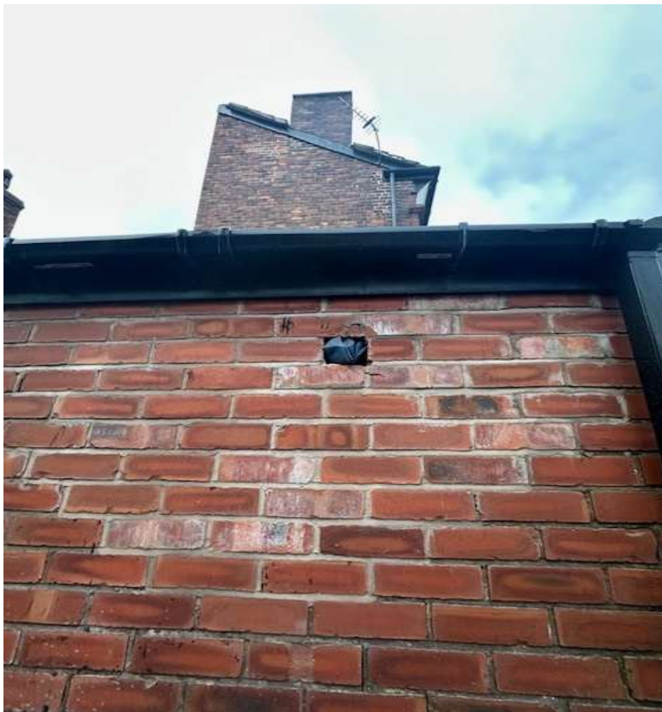
Figure 8: Partial removal of existing brickwork evidenced on the side elevation of the application property (garage).
