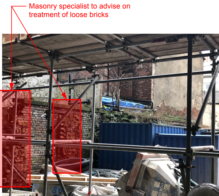
Wall F - Existing condition looks to be in poor condition visually. Key constraint is Booz 4 U boundary
