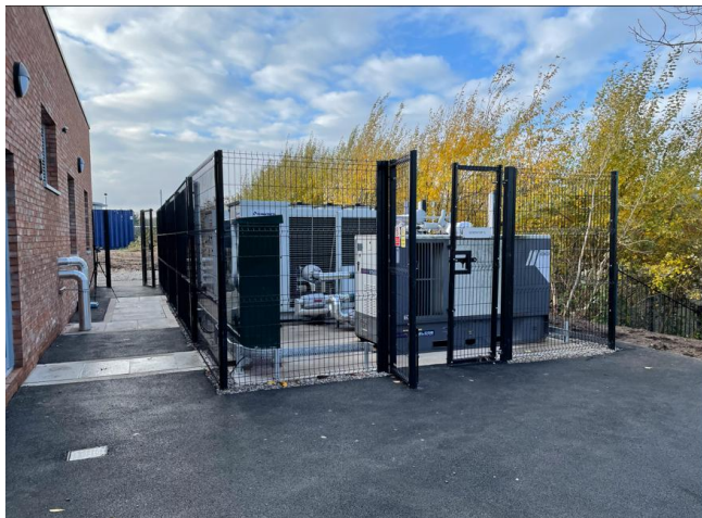
Figure 3 Photographs of the installed ASHP
