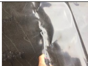
Recorded hand weld defect
