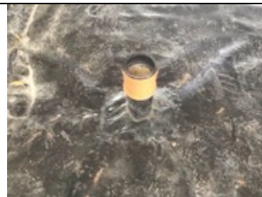
Sealed pipe penetration
