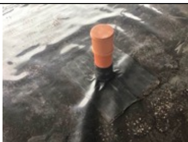
Sealed pipe penetration
