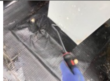
Pick testing stanchion sealing
