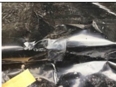
Recorded weld defect repair
