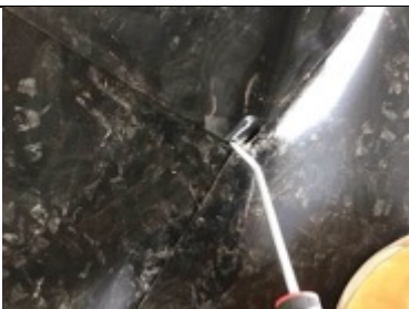
Recorded weld defect
