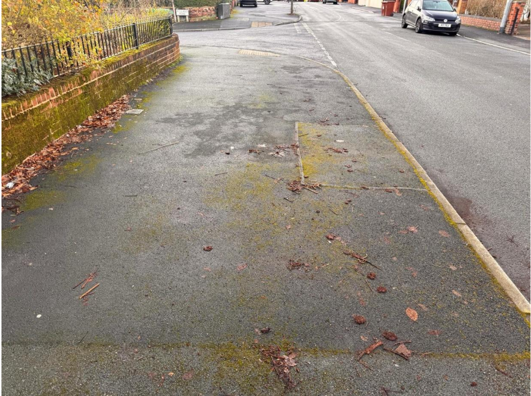
Figure 3: Pavement adjacent to Wilton Road, facing west. This shows a rectangular section of pavement (utility patch) which has been relaid.
