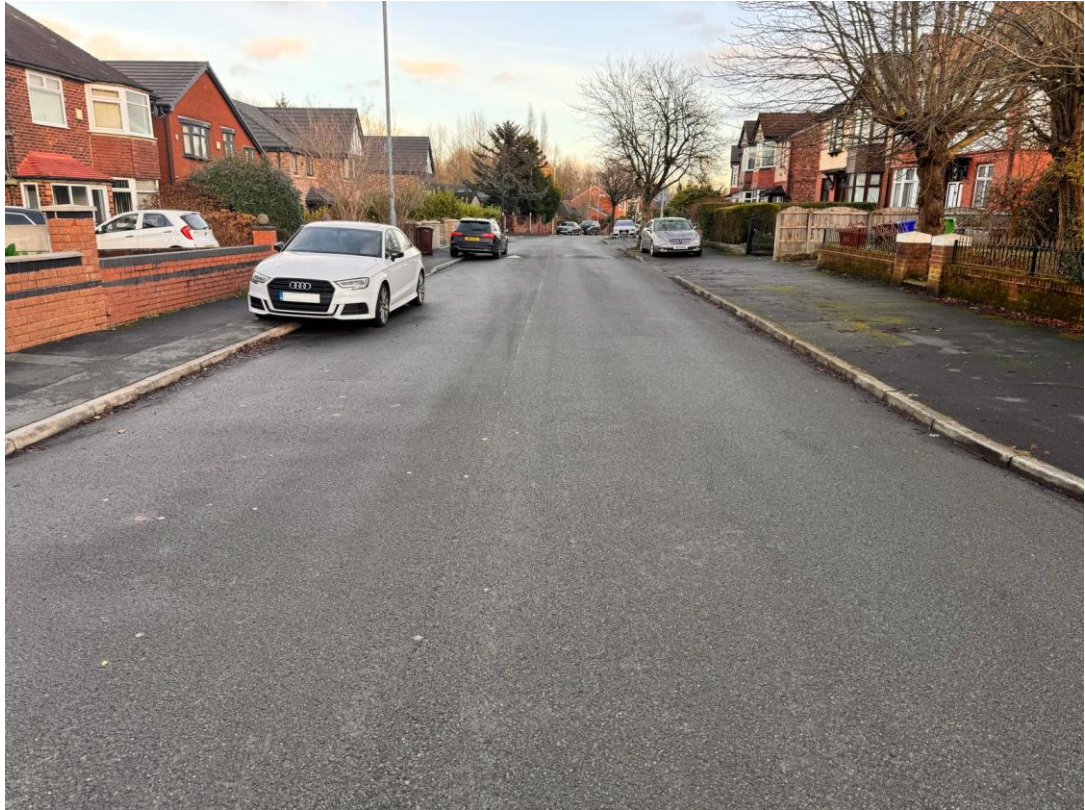
Figure 5: Wilton Road, facing east. This illustrates the existing staining of the kerbstones.
