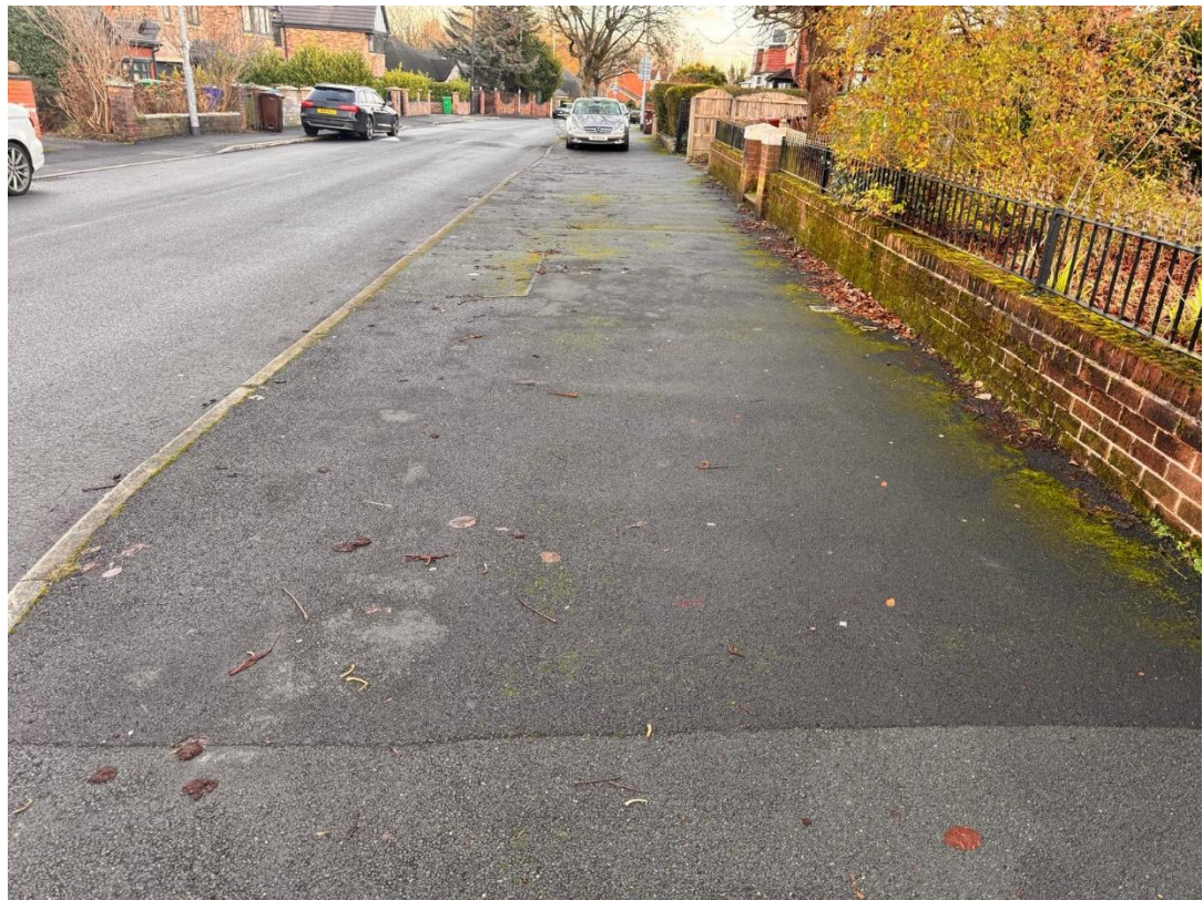
Figure 4: Pavement adjacent to Wilton Road, facing east. This shows that a large irregularly shaped section of the pavement has been relaid.
