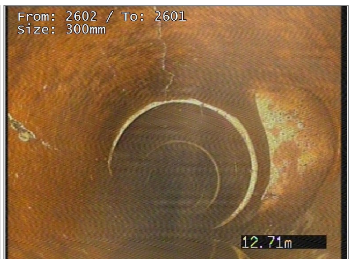
Fracture longitudinal at 8 o'clock
