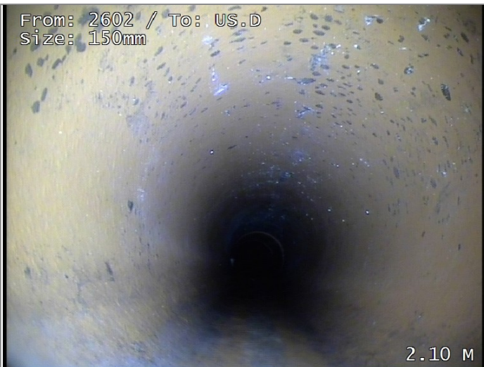
Joint displaced medium
