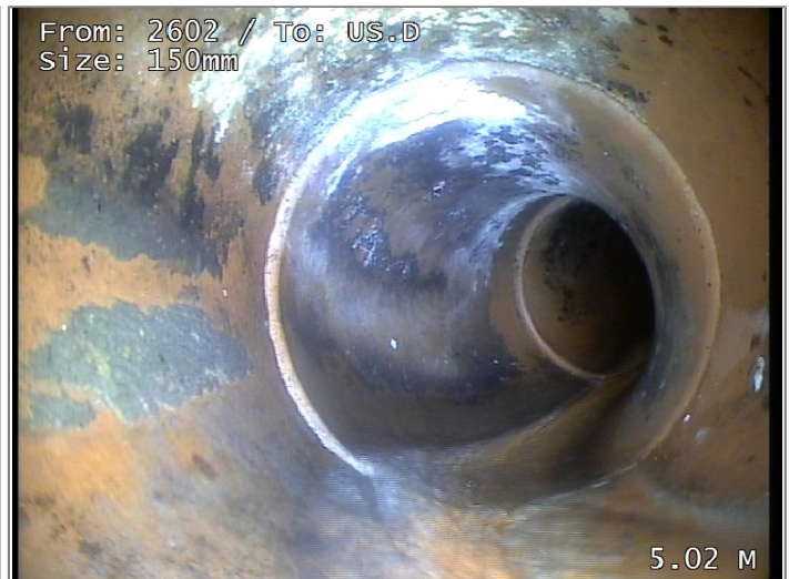
Line of drain/sewer deviates right
