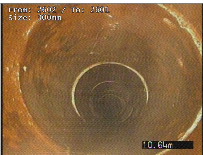
Fracture longitudinal at 12 o'clock, Start
