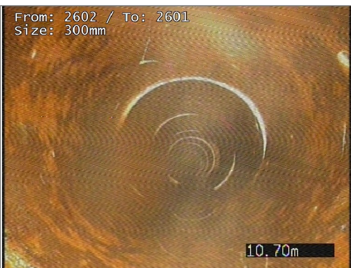
Fracture longitudinal at 12 o'clock, Start
