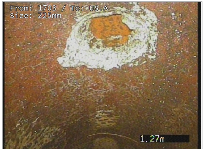
Spalling at 12 o'clock
