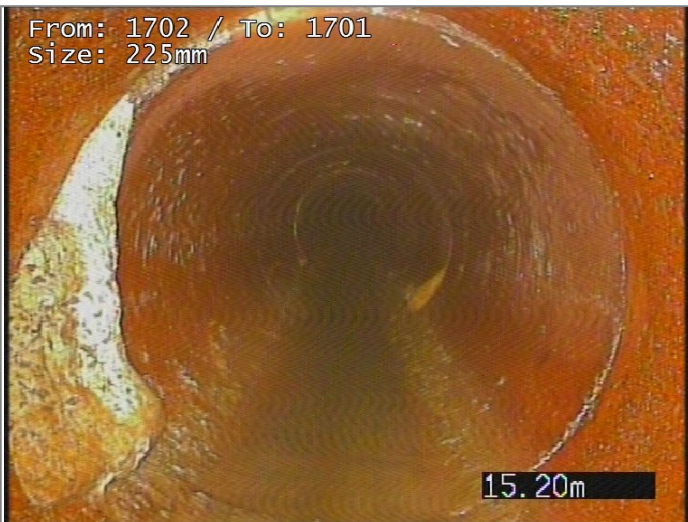
Other attached deposits from 7 to 11 o'clock 10% cross-sectional area loss - Remark CONCRETE, at joint
