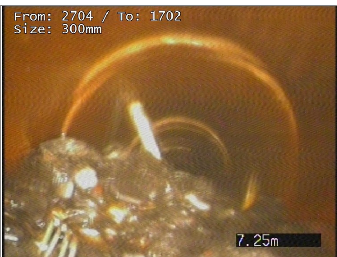
Settled deposits hard or compacted 50% cross-sectional area loss
