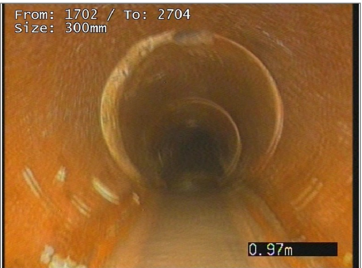
Crack circumferential from 2 to 10 o'clock
